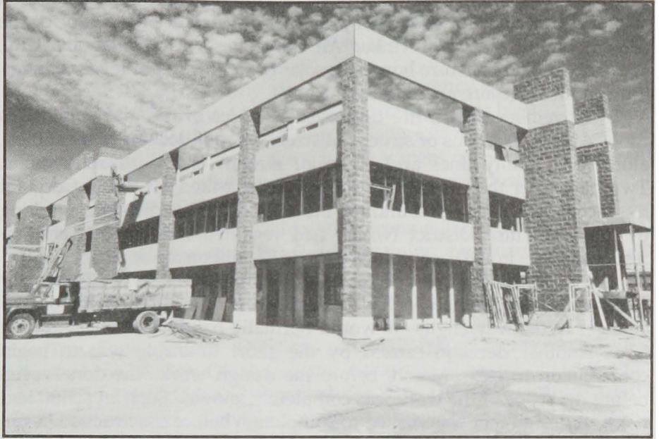
Enlisted-personnel barracks at Holloman Air Force Base, New Mexico, got a facelift and interior renovation through division efforts.
