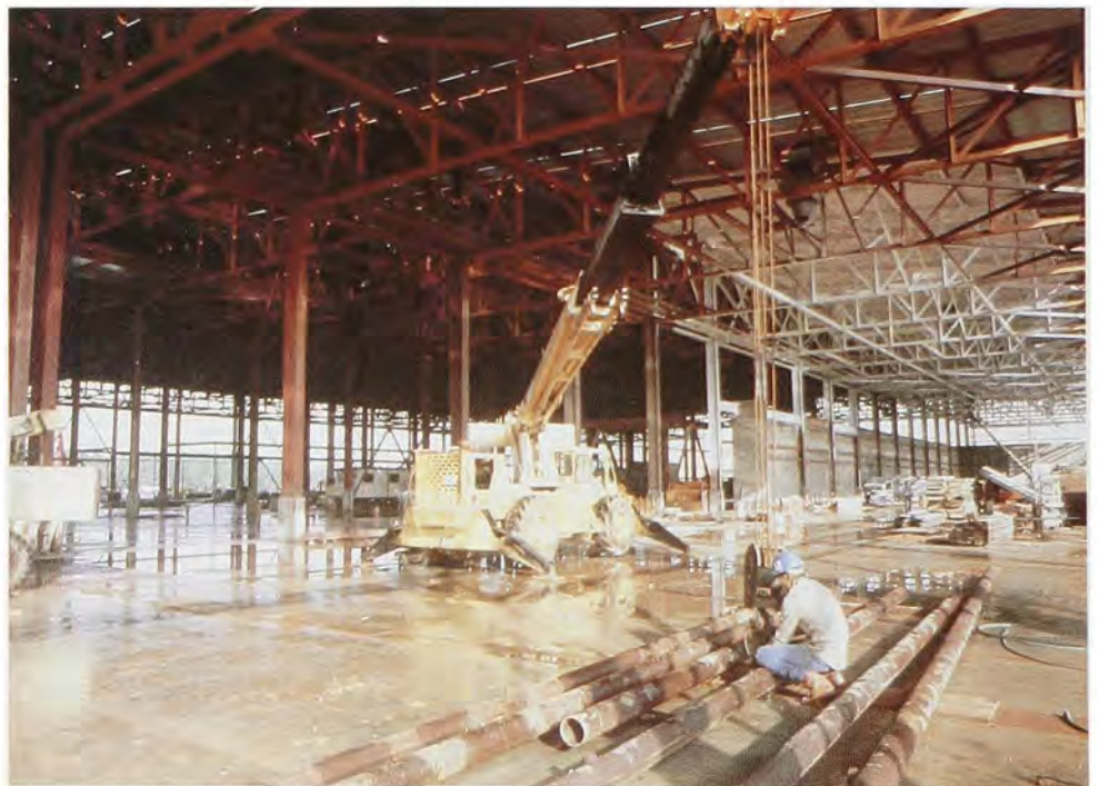
A crash program spearheaded by Southwestern Division and Air Force officials reconstructed the damaged Building 3001 at Tinker Air Force Base in ten months.
