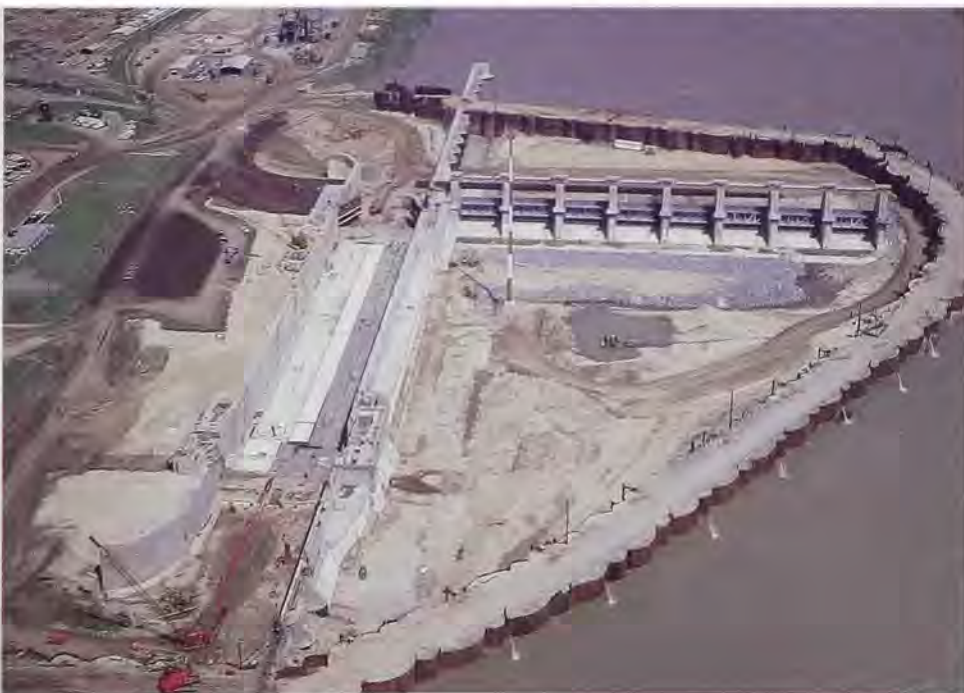
Construction at Lock and Dam No. 4 near Pine Bluff, Arkansas, made up one part of the McClellan Kerr-Arkansas River Navigation System.
