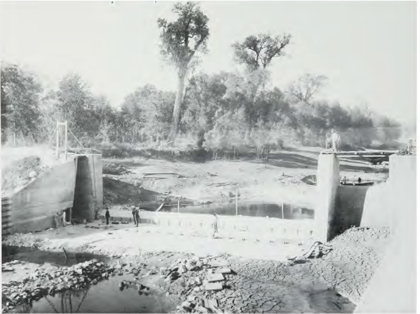
Workers labor at partially finished Lock and Dam Number 1 on the Trinity River near Dallas on 30 Oct. 1917. (Reprinted with permission of the Dallas Historical Society.)
