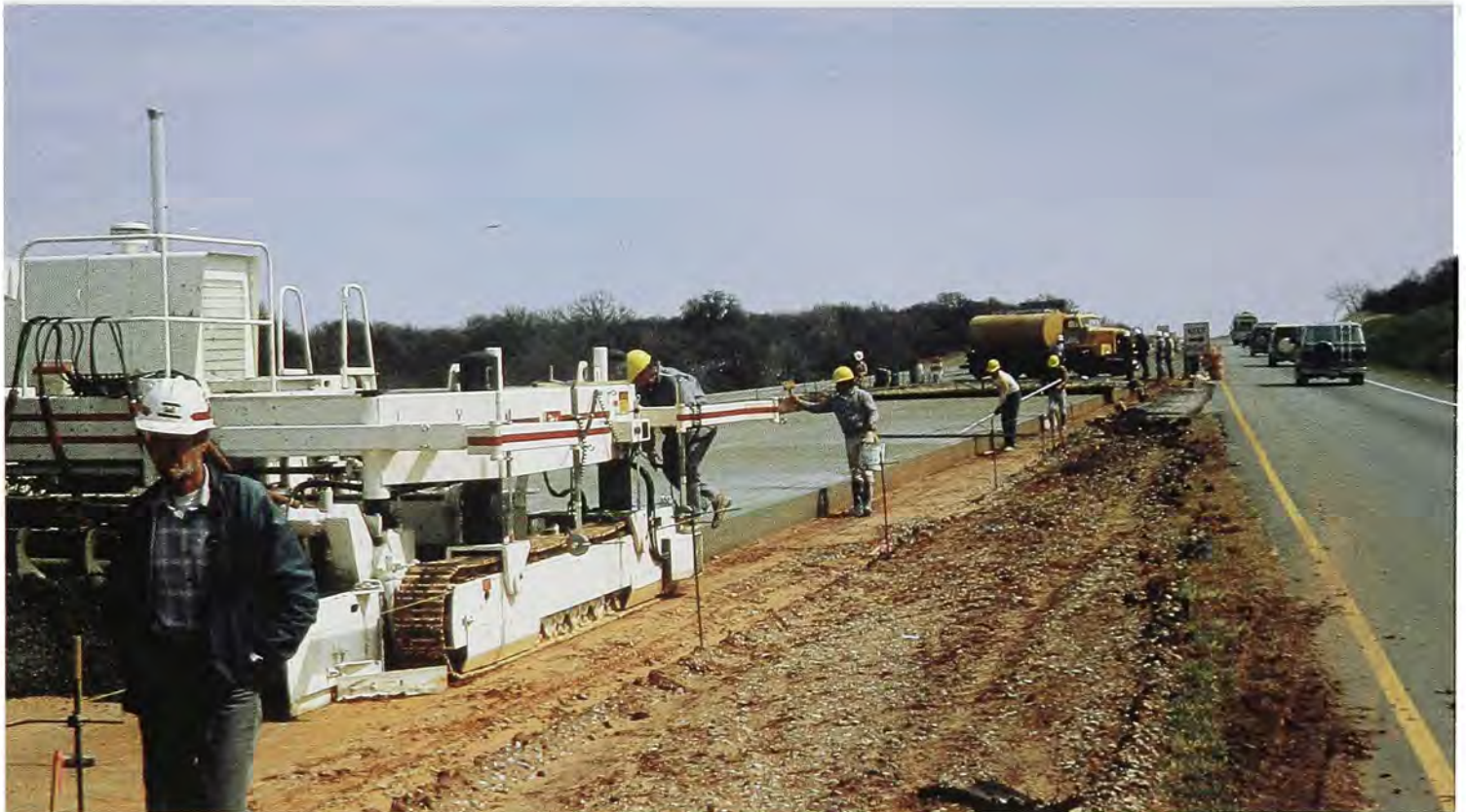
Workers relocate Turner Turnpike at Arcadia Lake as construction nears completion in 1986.
