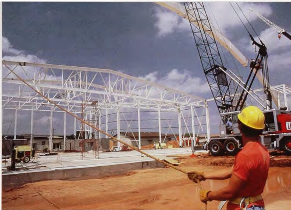
This hangar and other facilities built by the Fort Worth District at Dyess Air Force Base, Texas, house the Air Force's first operational B-1B squadron.
