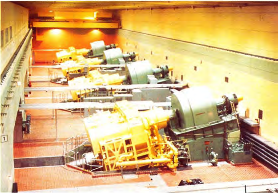
Slant-axle turbines in the Ozark powerhouse on the Arkansas River.
