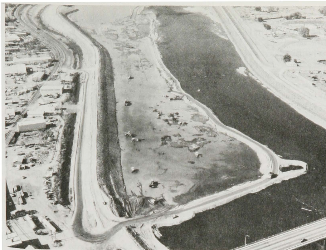
CLEARWATER RIVER - MEMORIAL (16TH STREET) Bridge Downstream - Levee and By-Pass Road Along Lewiston Waterfront Holbrook Island Excavation Center of Picture North Bank Levee in Place
