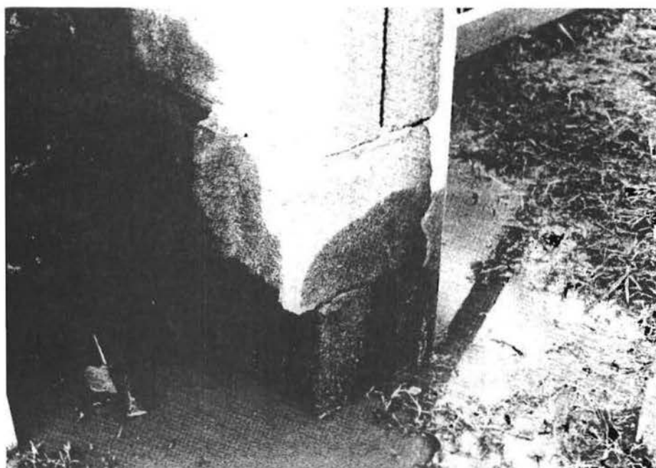
b. Base of wall
