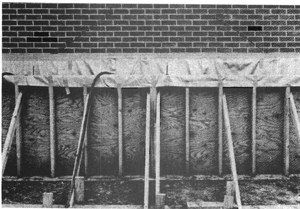
Figure 10. Wall 1. Failure pattern of wall
