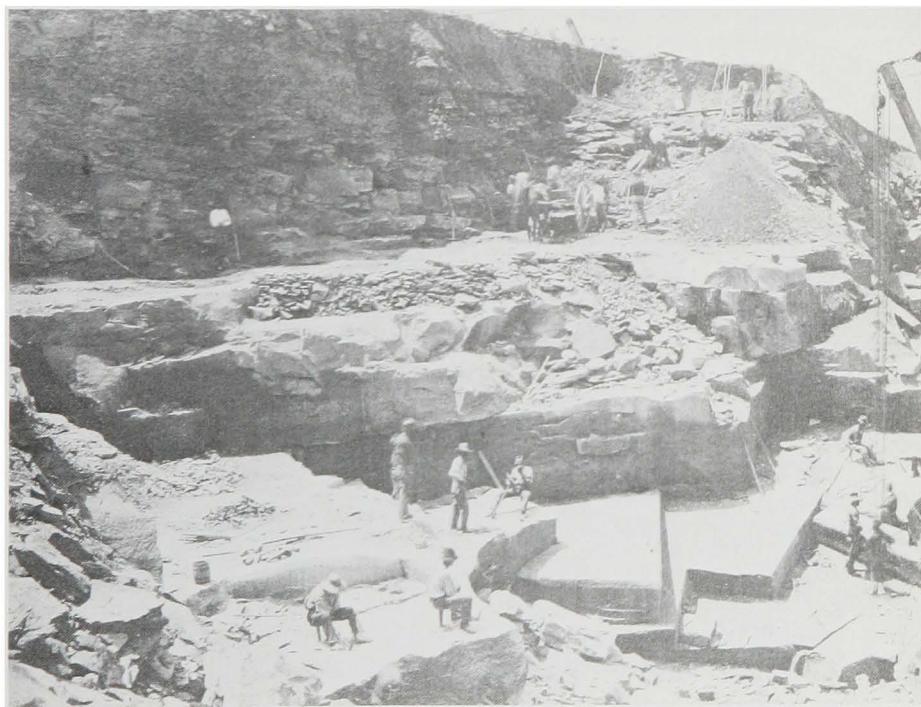
Quarrymen cutting the stone to be used in the Davis Island Lock. The derrick at the right is preparing to lift one of the dimension stones.
