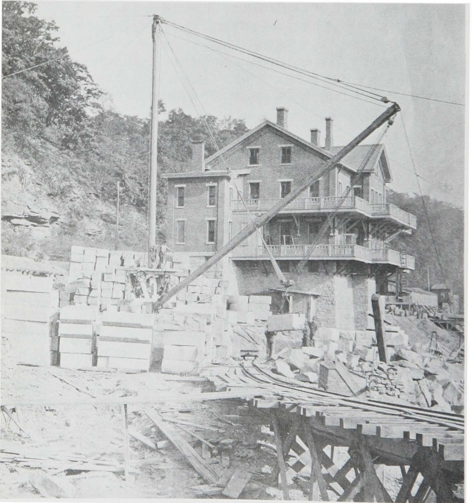
A stiffleg derrick lifts a stone for placement atop the rail car and movement to the lock’s land wall. The completed lock house is in the background.
