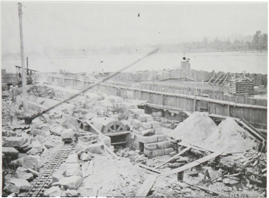
A rail car carrying a stone arrives under a stiffleg derrick, which raised the stone for placement in the lock wall next to the filling and emptying culvert.
