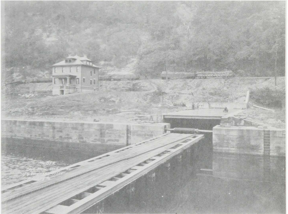
This picture of the rolling lock gate at Ohio River Dam 6 shows the drum and chain used to move it in and out of its recess. In the background is the lock house and several car loads of construction materials.
