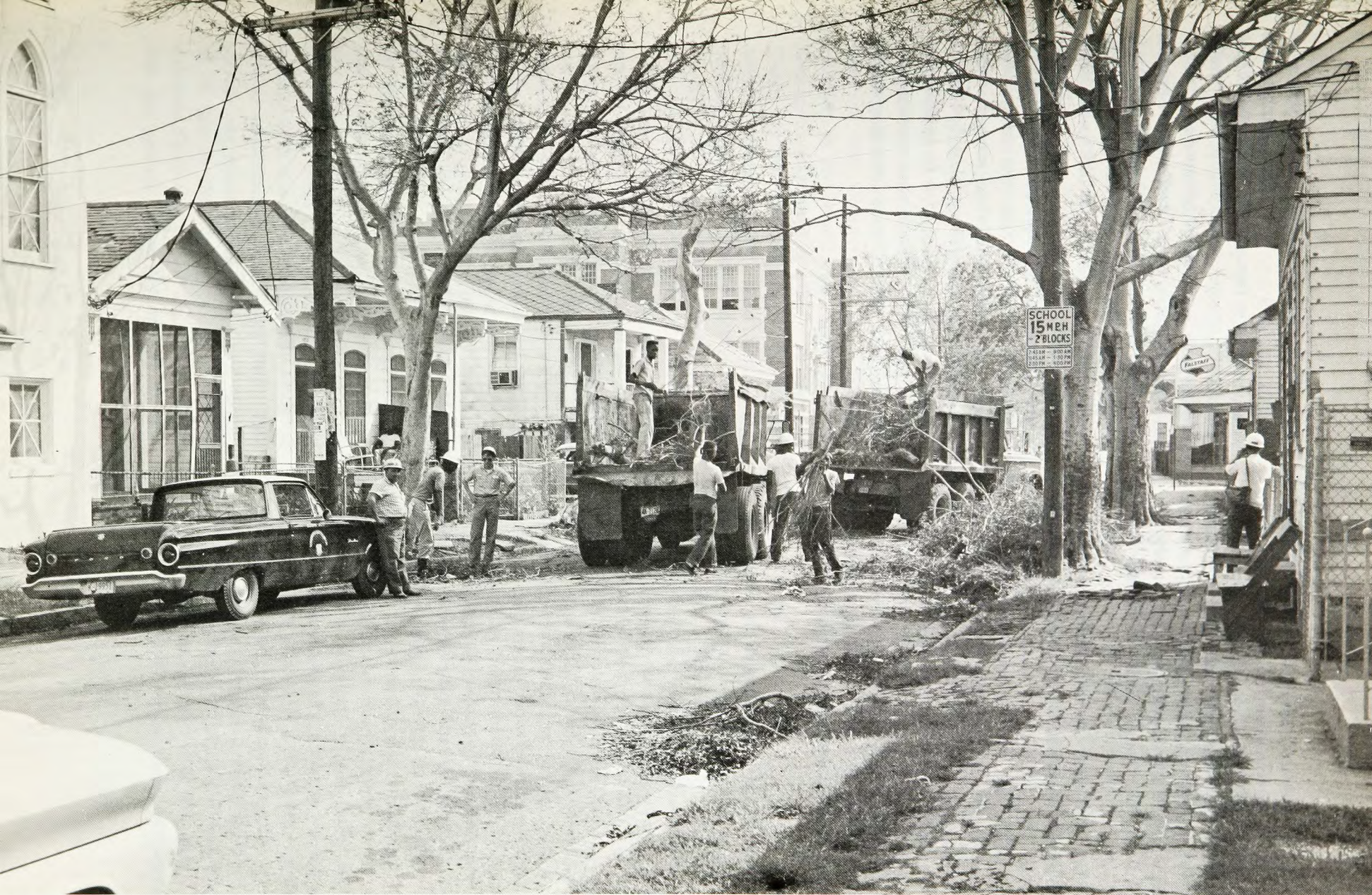
Fig. 15. The cleanup job – a new responsibility for the New Orleans District. New Orleans, 1965.
