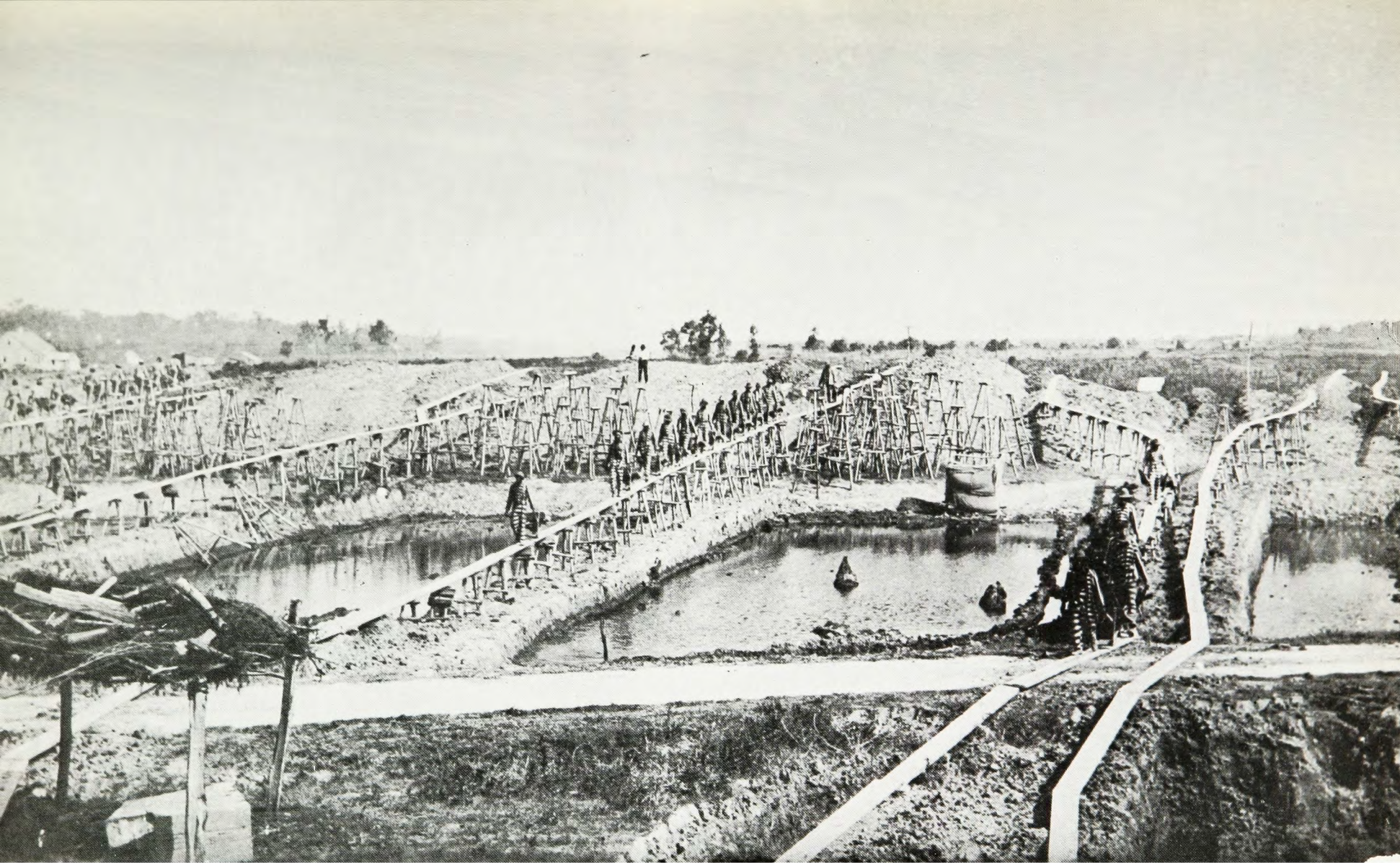
Fig. 3. Levee building — old style. Convict and free labor work side by side at the Morganza crevasse, 1890. (Photographer unknown)
