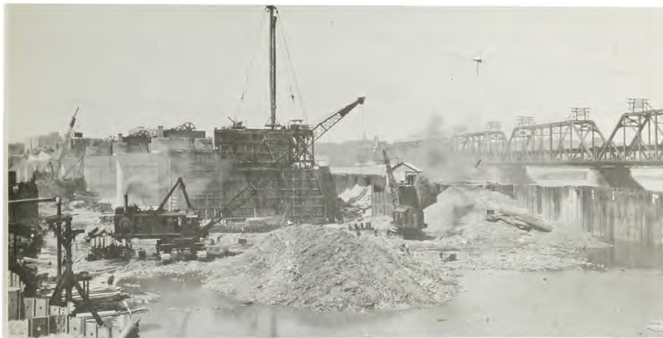
Construction on Dam 15 at Rock Island shows its location just downstream from the Rock Island Bridge. Lock 15 utilizes the original drawspan of that bridge.
