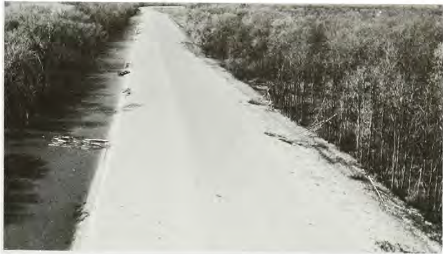
High water conditions in the Muscatine Island Levee District showing a typical rural levee system at work.
