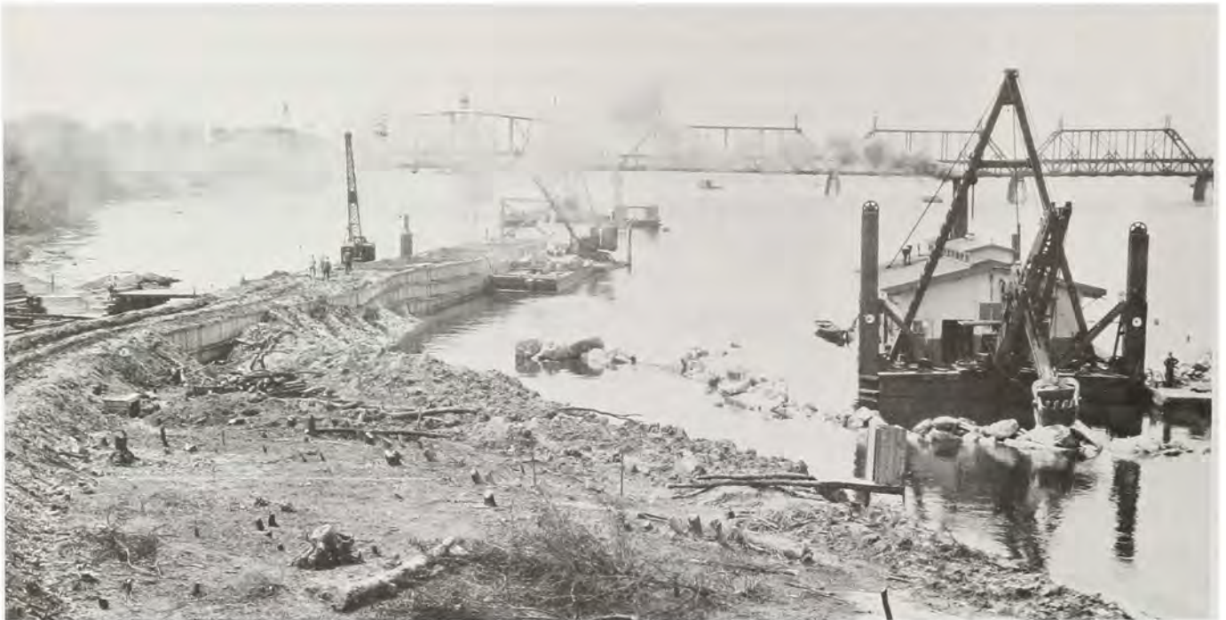
Initial construction on the 9-foot channel began with this coffer dam at Lock 15, adjacent to the new headquarters of the Rock Island District.
