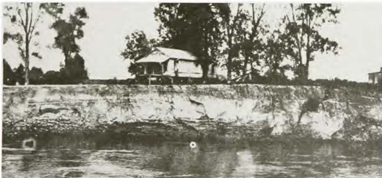
Bank caving on the Mississippi threatens nearby tenant house
