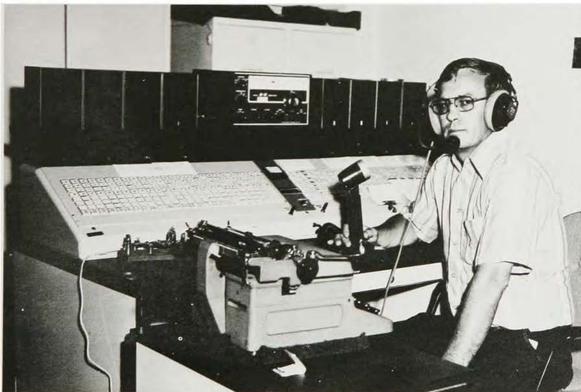
This radio component system features mobile dispatch and telephone patch, telegraph, and the capability to tune the receiver-antenna automatic caller over 6 miles away. This setup, of which there are three, was built in the District's Electronics Shop
