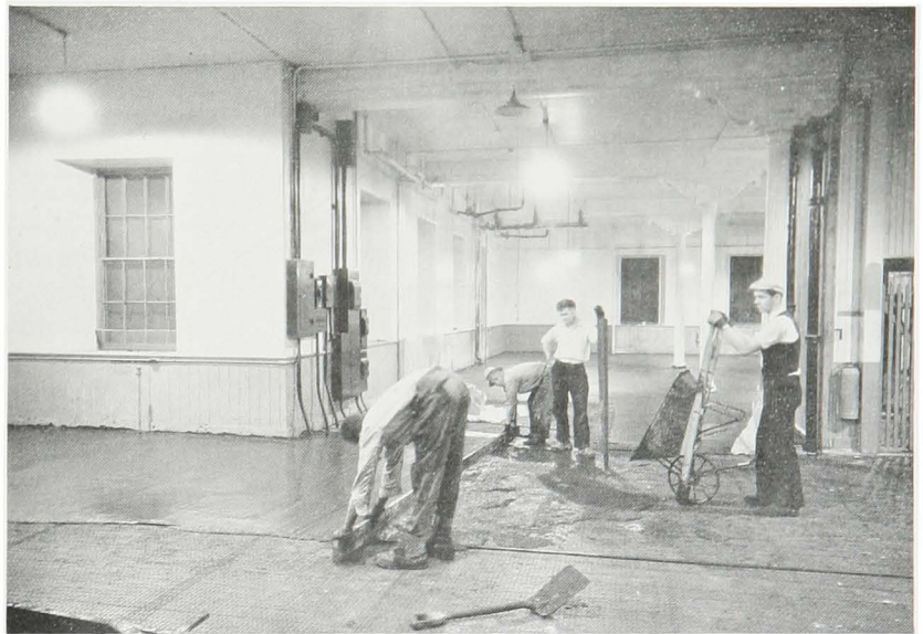
Fig. 20. Plastic mortar being placed between wooden screeds during resurfacing of the third floor in 1935.
