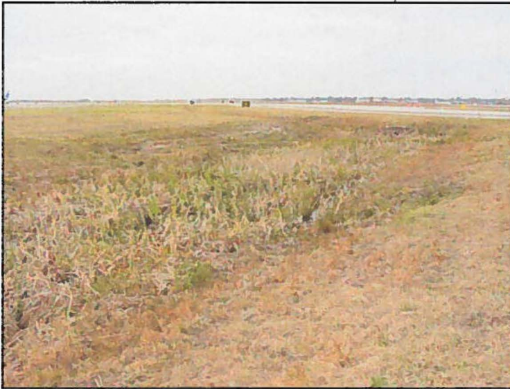
Runway 21, cleared safety zone to be graded as part of the 1,000 by 2,000-foot graded cleared area.
