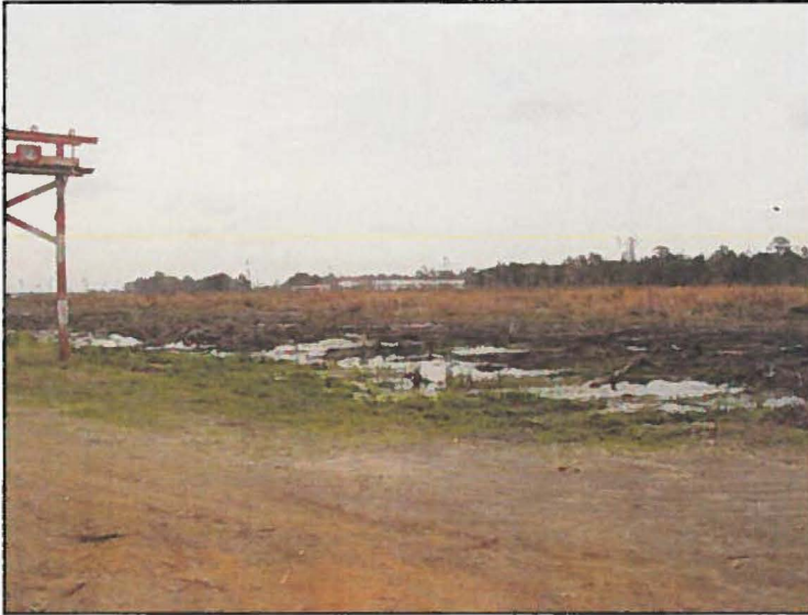
Runway 03, cleared safety zone to be graded as part of the 1,000 by 2,000-foot graded area.
