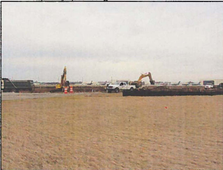
Stormwater facilities work being conducted in Fall 2004, as runway 21 as part of a separate project.
