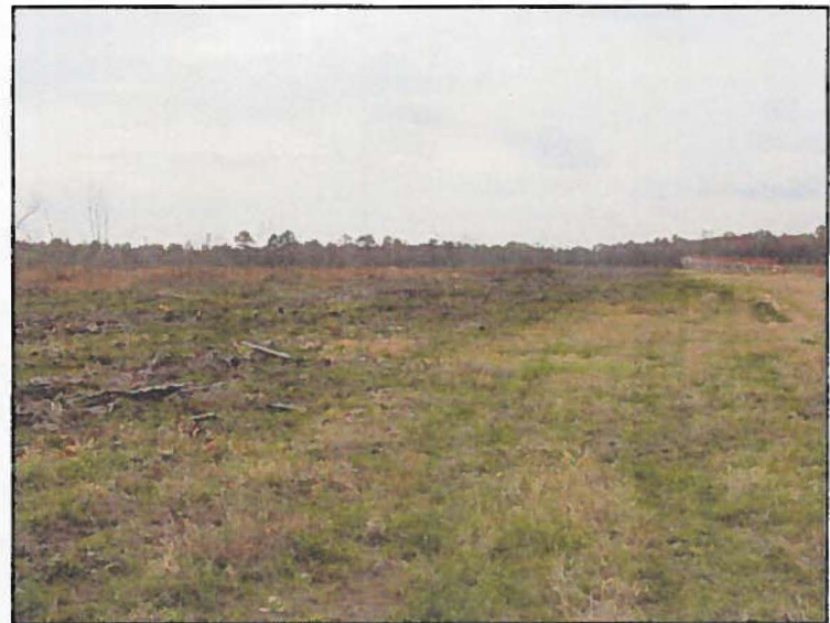
Runway 03, cleared safety zone to be graded as part of the 1,000 by 2,000-foot graded area.
