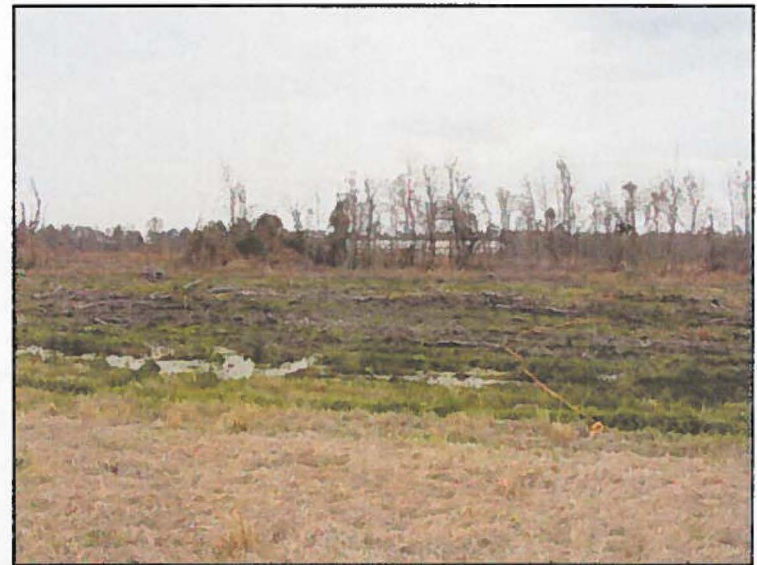
Runway 03, cleared safety zone to be graded as part of the 1,000 by 2,000-foot graded area.
