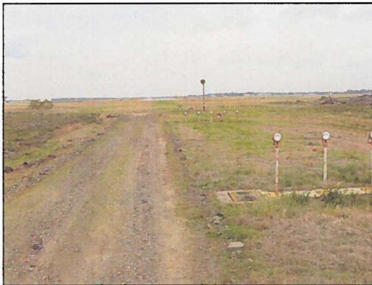
Runway 03 facing north, cleared safety zone to be graded as part of the 1,000 by 2,000-foot graded area.
