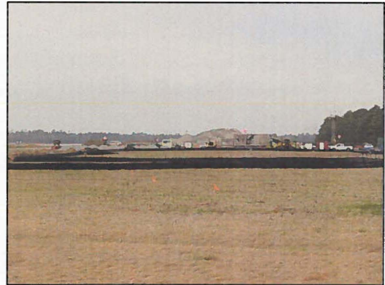
Runway 21, existing cleared safety zone to be graded as part of the 1,000 by 2,000-foot graded cleared area. Current work being conducted.
