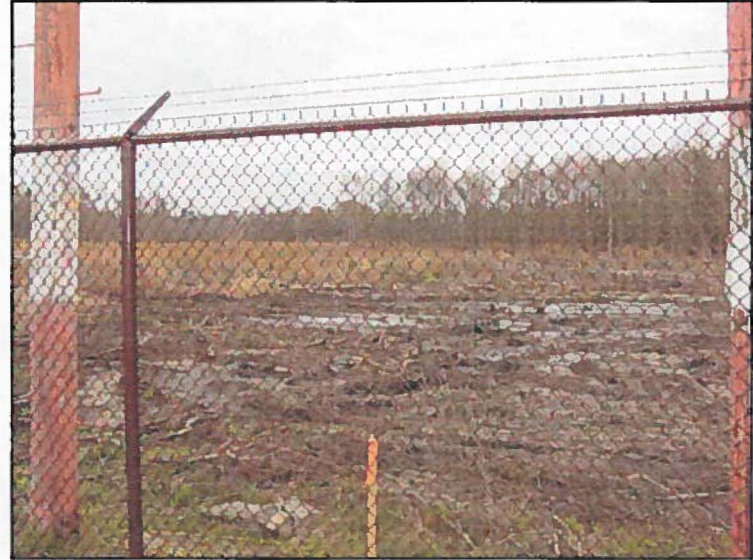
Runway 03, cleared safety zone to be graded as part of the 1,000 by 2,000-foot graded area.
