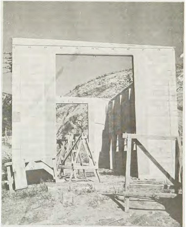
Defaulted maintenance building, TAC Site
