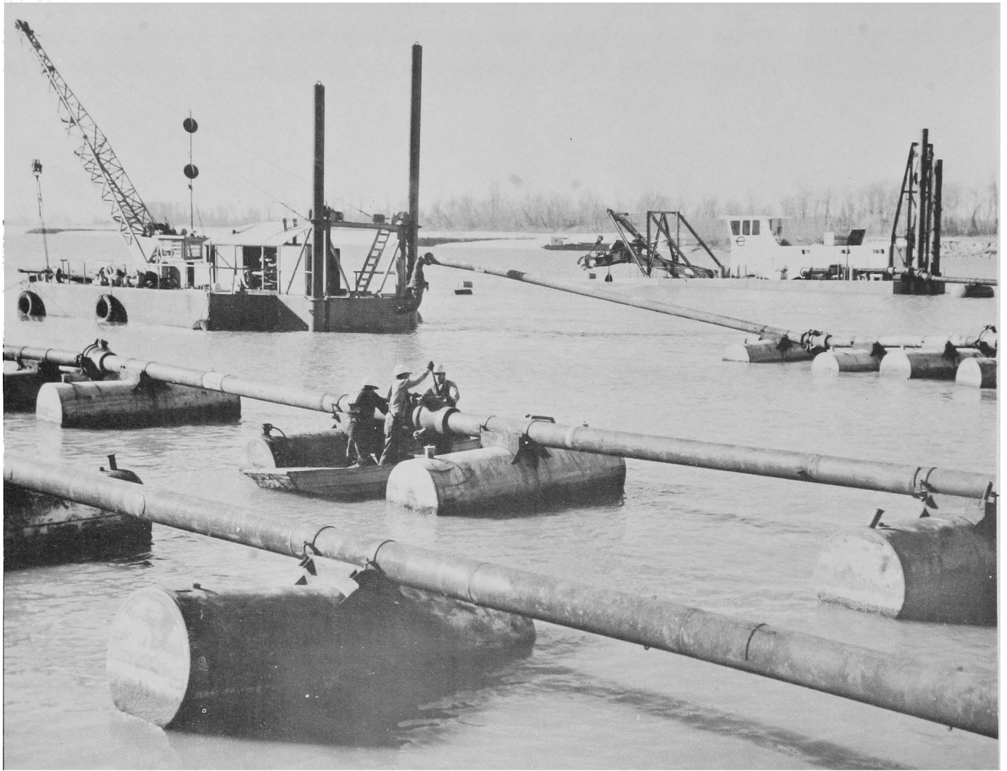
Large suction dredges remove shoals from Arkansas River Navigation Channel below Toad Suck Ferry Lock & Dam near Conway, Arkansas.
