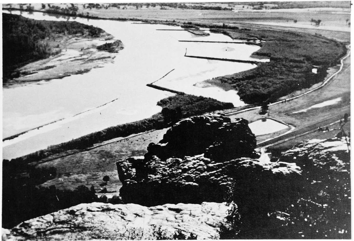
Bank Stabilization on the Arkansas River keep the meandering river within stable bounds.
