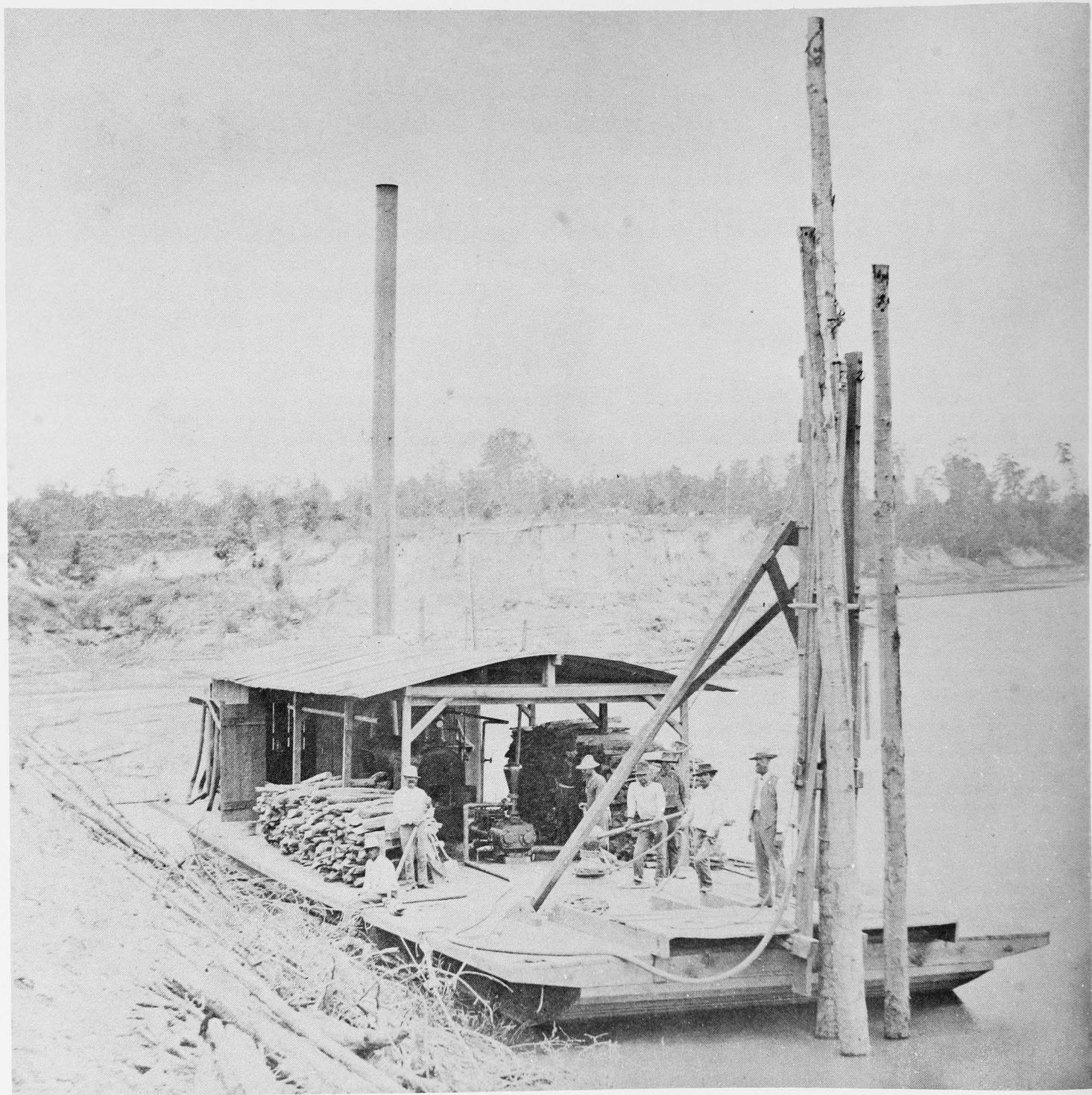
Hydraulic pile-driving on the Arkansas River at Pine Bluff, Arkansas in 1881, the year the Little Rock District was formed.
