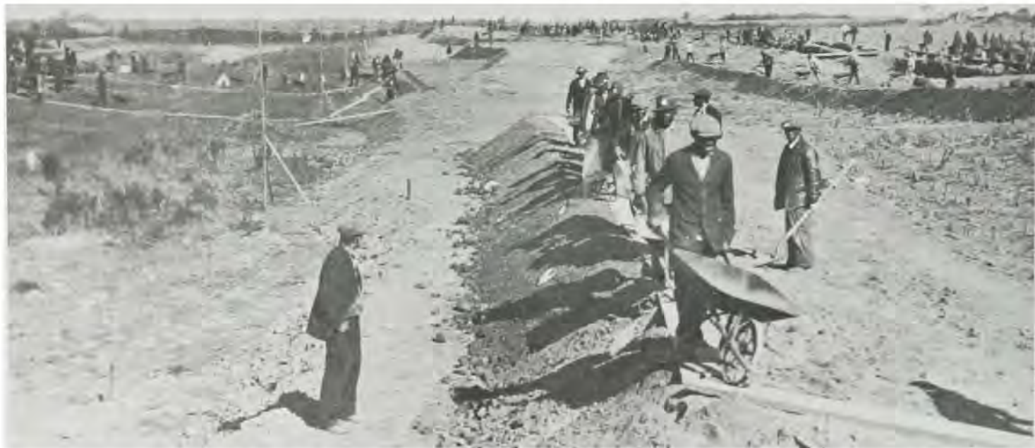
Workmen employed under the Emergency Relief Appropriation Act moved earth with hand tools on the embankments of the Chesapeake and Delaware Canal.
