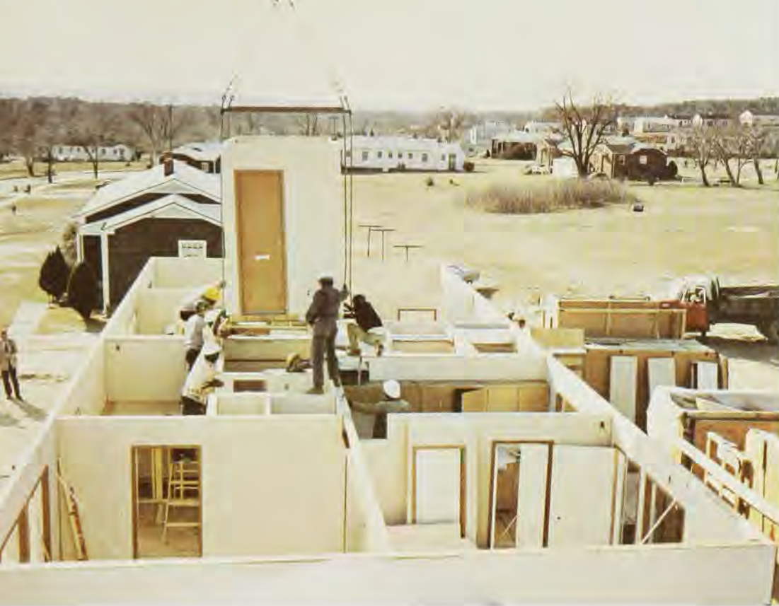
USAHOME — Modular second floor core being lowered into place, with all first floor panels in position. Proficient technical work crews could rapidly assemble the prefabricated coded units, on masonry foundations laid by other workers at locations throughout the world.
