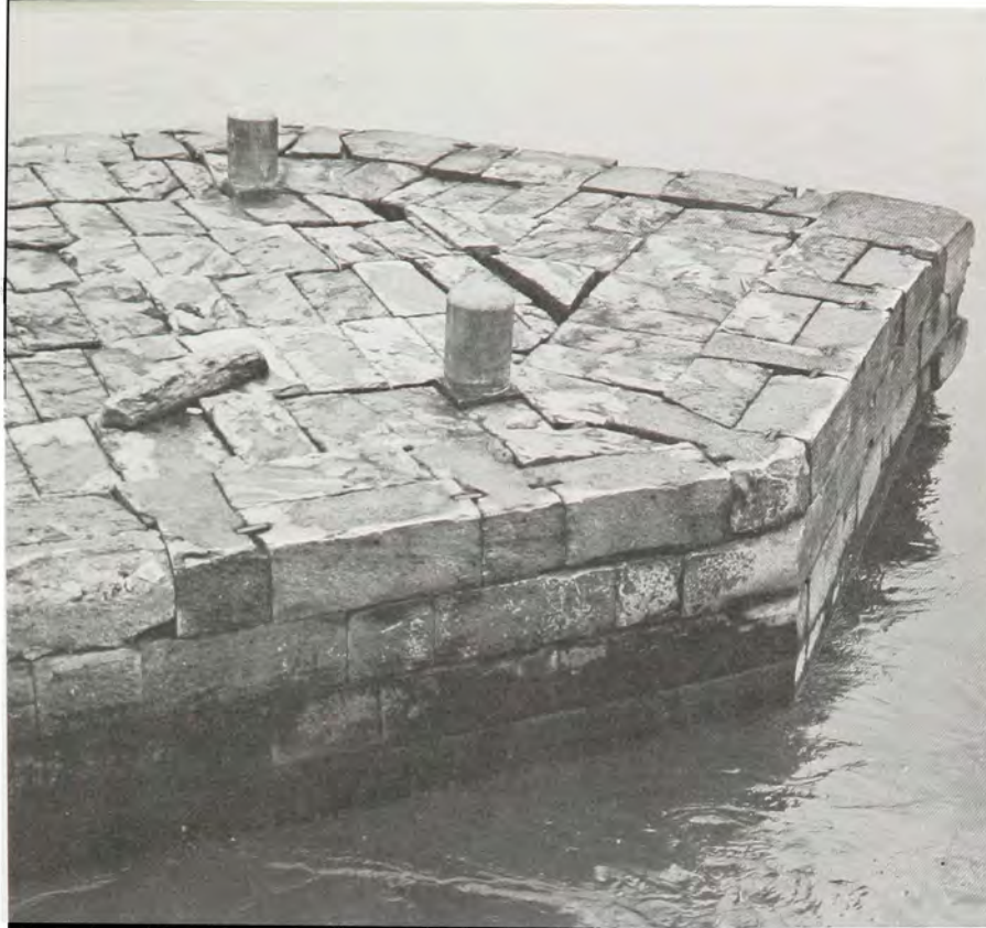
Typical top course features are the mooring posts, butterfly key headers and wrought iron ties for the outside stones.
