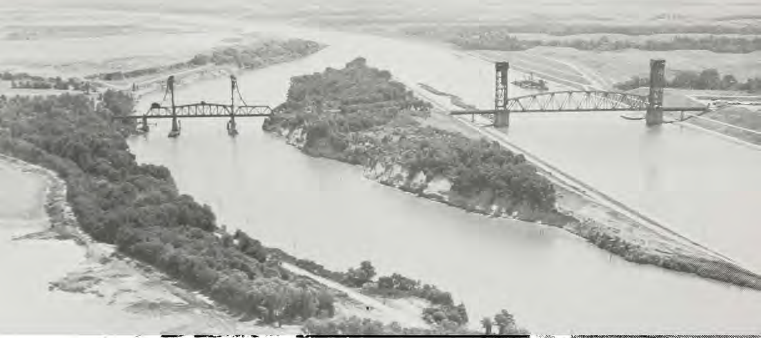
Nearing completion in this 1968 view is the cut-off channel with new railroad lift bridge. This improvement eliminates the navigational hazards of Lorewood curve and the narrow span at left.
