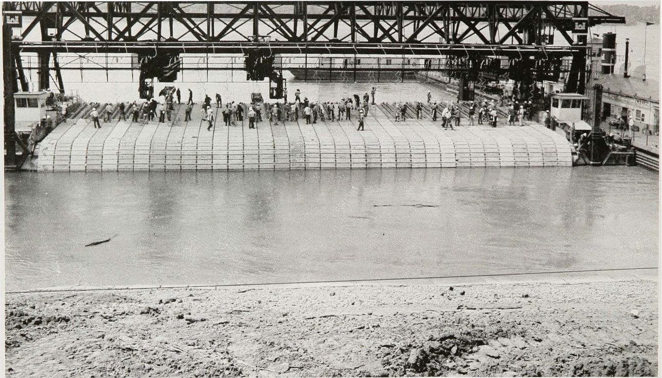
Newly formed rows of the concrete mattresses slide off the sloping deck onto the bank.
