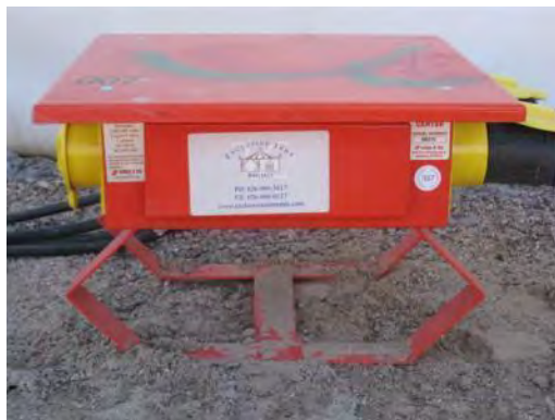
Heater Power Dist. Box
