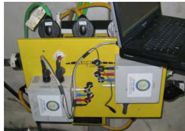
Tent Power Dist. Box
