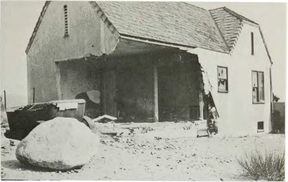
House on east side of flood channel between Prospect Ave. and Evelyn St. damaged by flood water and debris (Jan. 1, 1934).
