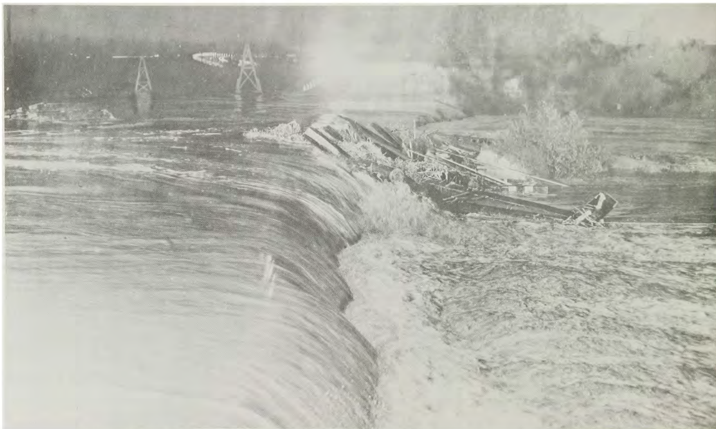
Destruction of the Beverly Blvd. crossing on the San Gabriel River, Calif. (Flood of January 15-18, 1952.)
