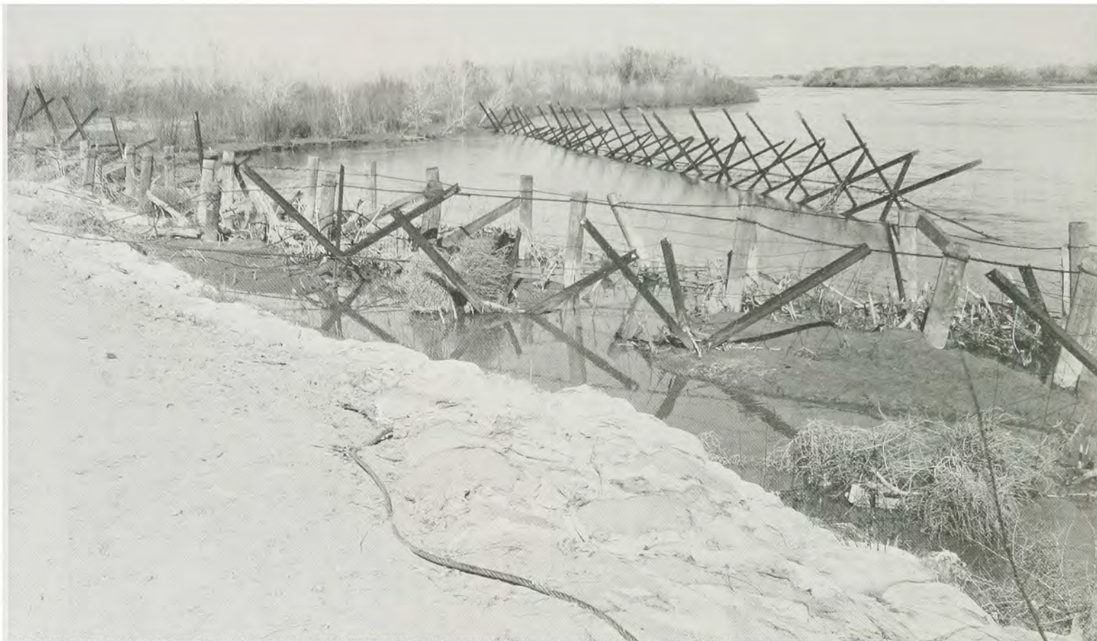
Plate No. 32. Local Flood Protection on the Rio Grande near Corrales, New Mexico
