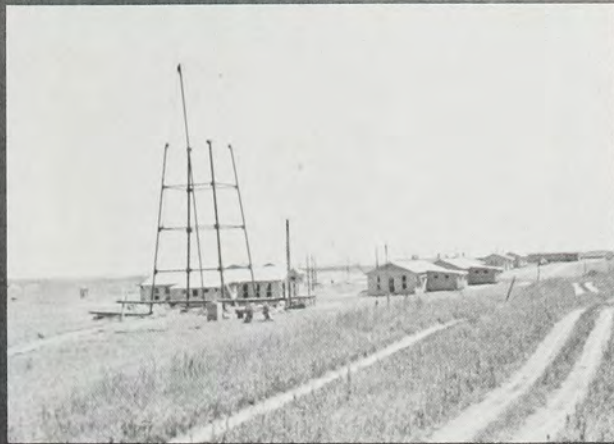
Keystone Dam penstock dwarfed workers, 1960. Top left, Fort Gibson concrete work, 1917. Top right, laying water line, Great Salt Plains Dam, 1938.
