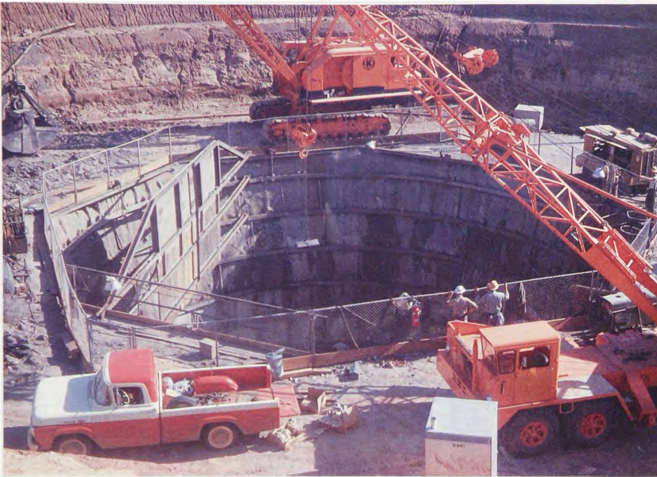
There was nothing simple about building the intricate Atlas missile facilities near Altus in the early 1960s, one of the greatest military challenges ever faced by the Tulsa District.
