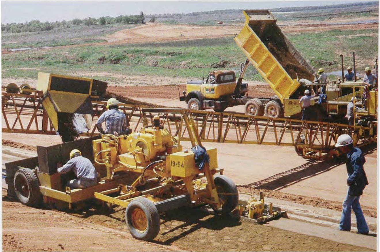
Top left, construction geared up in 1982 for Arcadia Dam near Oklahoma City, while Copan Lake near Bartlesville opened in 1983. Equipment called a "mole" tunneled through the Osage Hills to help complete Skiatook Dam in 1984.
