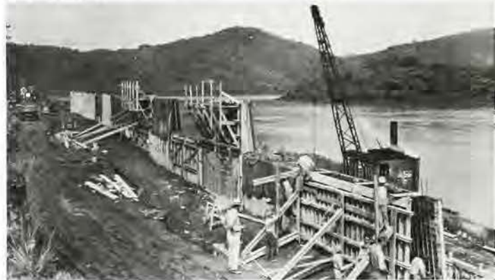
Construction Crew building the flood wall to protect Sunbury, Pennsylvania, July 14, 1948. U.S. Army Corps of Engineers—National Archives
