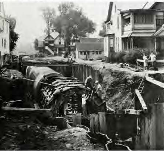
Conduit construction in Elmira, New York, August 8, 1947. U.S. Army Corps of Engineers—National Archives
