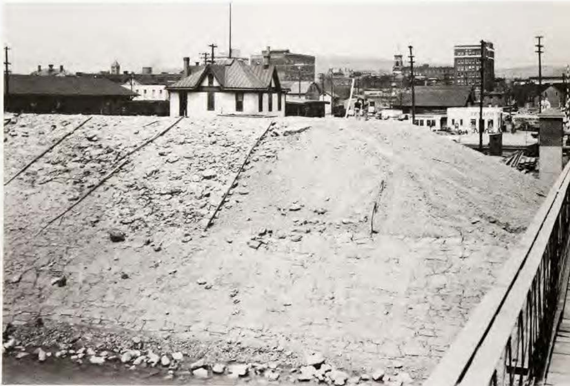
Levee embankment with partially completed rock paving at Williamsport as it appeared on May 12, 1948. U.S. Army Corps of Engineers—National Archives
