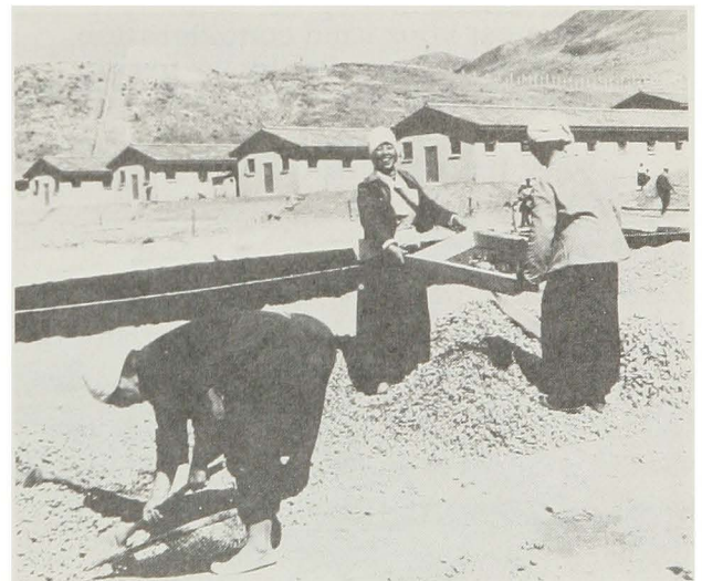
Korean women laborers screening aggregate for road construction at Taejon, Korea, in 1960. Compare this method of aggregate screening with the equipment illustrated in the 1969 photograph of the Suwon batch plant on page
