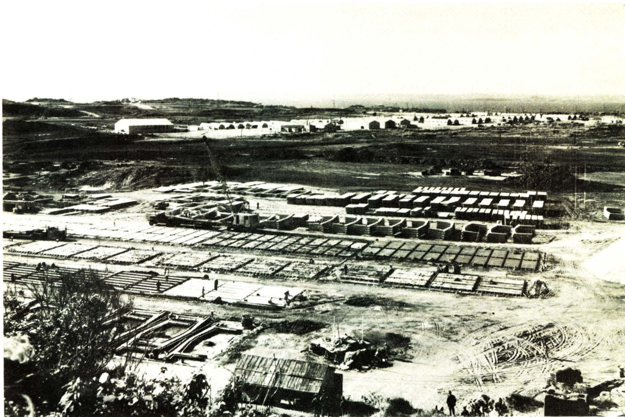
View of Kokuba Gumi's precast concrete yard installed at the construction site of Camp Hansen, Okinawa, in the early 1960's.
