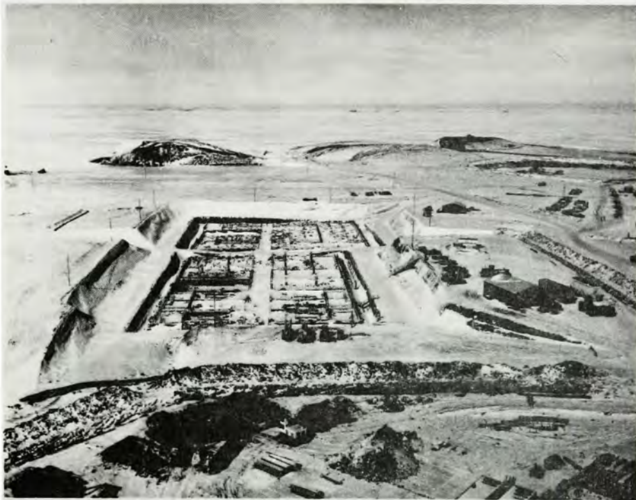
THE MSR SITE being constructed near Conrad, Montana, as part of the Safeguard BMD system, as it appeared in March, 1972. In the center foreground is the straw covered base slab of the power plant with the base slab of the MSCB immediately above.
