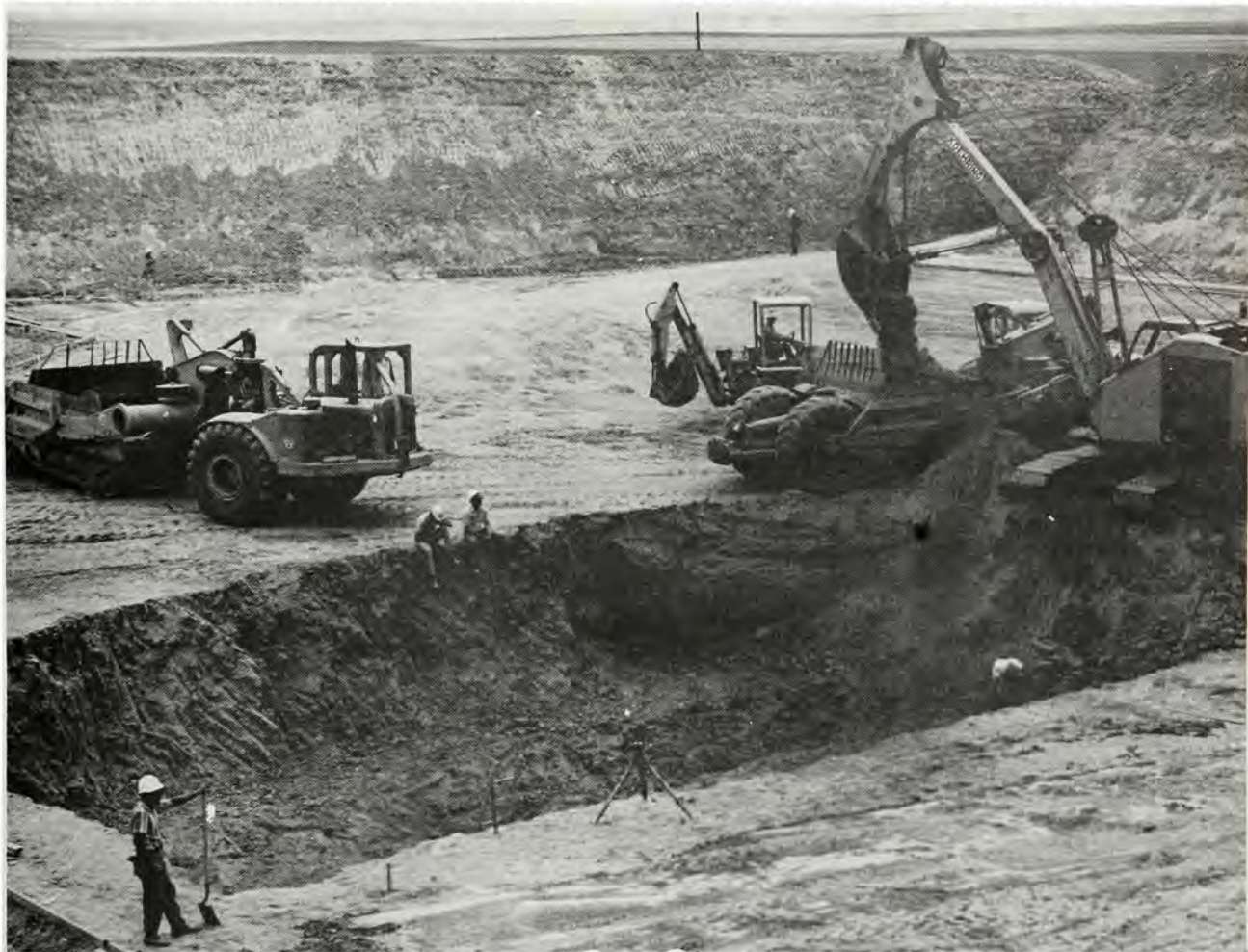
EXCAVATING FOR THE UNDERGROUND POWER PLANT of the Perimeter Acquisition Radar on July 10, 1970 at a site about 35 miles northeast of Conrad, Montana, as part of the Malmstrom Safeguard ballistic missile defense system complex. The work was under the supervision of the Malmstrom Area Engineer, Huntsville Division, US Army Corps of Engineers.
