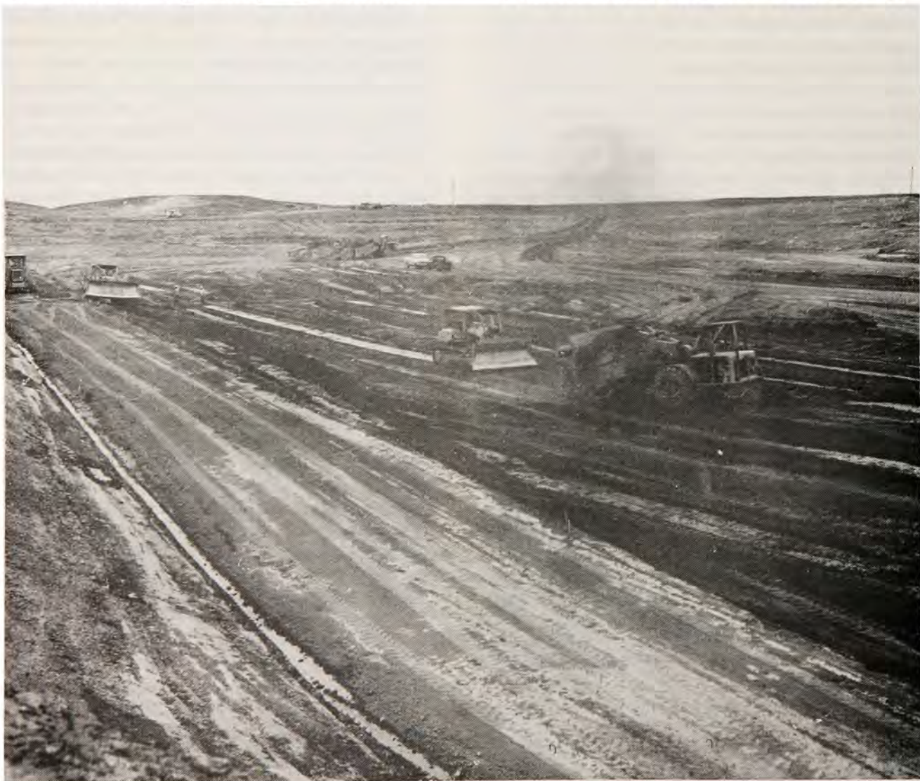
EXCAVATION UNDERWAY FOR THE MISSILE SITE RADAR BUILDING in July, 1970, as part of the Malmstrom Montana SAFEGUARD ballistic missile defense system complex.
