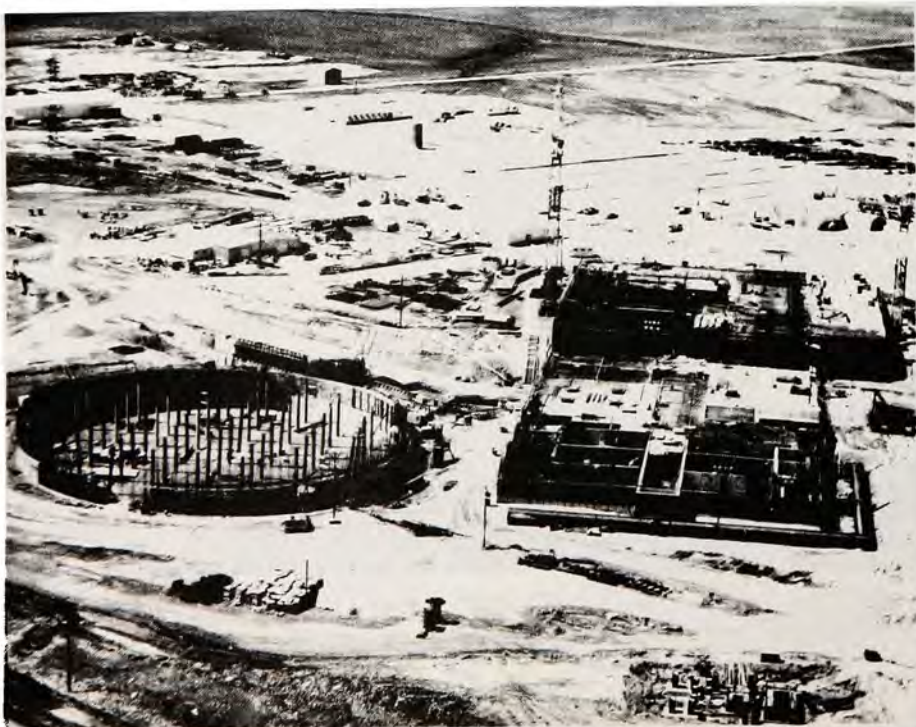
THE MISSILE SITE RADAR SITE in June 1971 during construction near Grand Forks. At left is the 7-1/2-million-gallon capacity heat sink which will be underground when completed. At right center is the 17.3 megawatt power plant with its roof being closed in. Directly behind the power plant is the Missile Site Control Building with the third floor structure being roofed in and the radar turret starting to be formed up.
