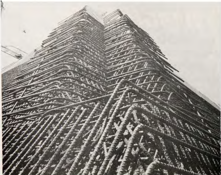
AN INTRICATE MASS OF REBAR FOR THE TURRET WALL of the nation's first Safeguard ballistic missile defense system complex at Grand Forks, North Dakota (July 1971).
