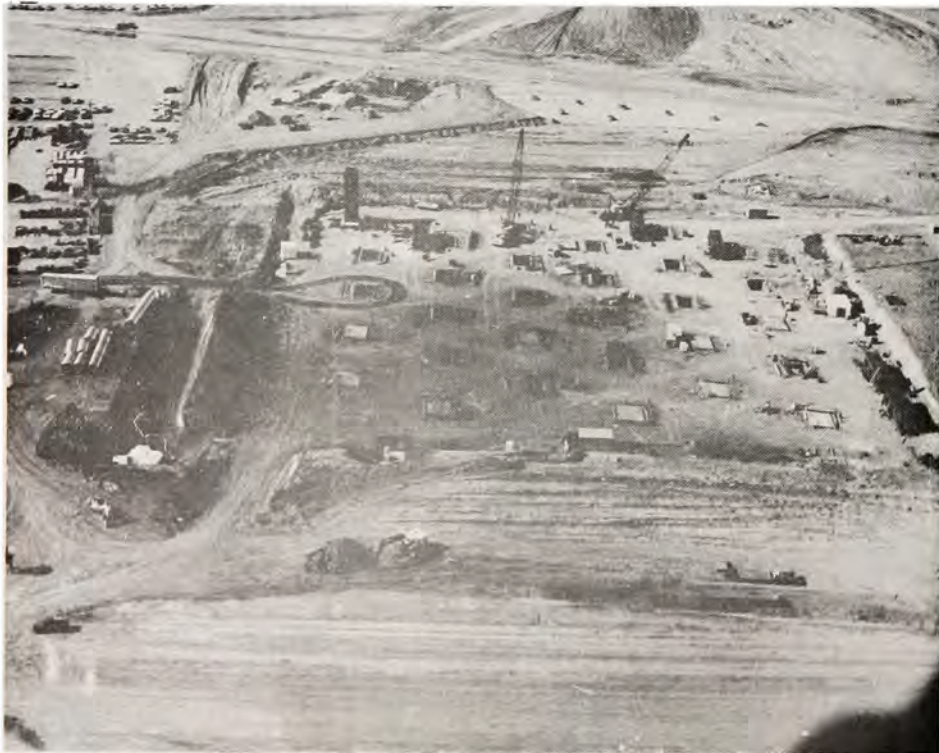
SQUARE HOLES FOR ROUND PEGS at the Spartan missile field of the Grand Forks SAFEGUARD BMD complex near Langdon, North Dakota, in October, 1970. The tall tower at the left rear of the field is a Spartan can surrounded by reinforcement steel. The unit will be lowered into one of the many square holes where it will receive concrete placement. The round Spartan missile will eventually be housed in the square reinforced concrete silo.
