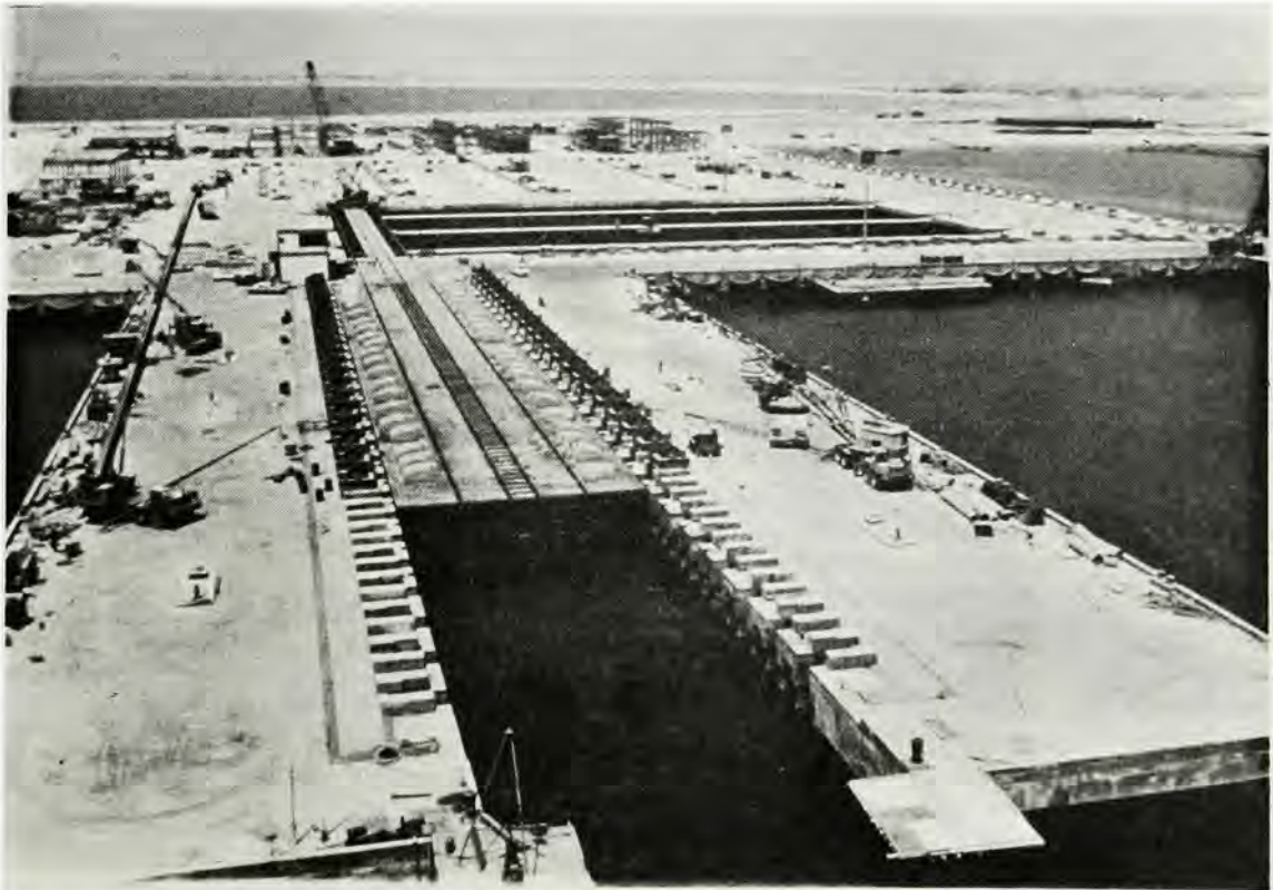
At Jubal, Saudi Arabia Piers 3 and 4 have a synchrolift.
