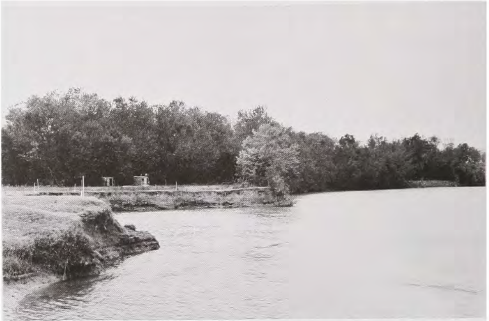
Canoe Cut on the Savannah River below Augusta before construction of bank protection work was begun by Leroy H. Simkins of the Corps of Engineers. 16 October 1940. (Savannah District, Corps of Engineers)
