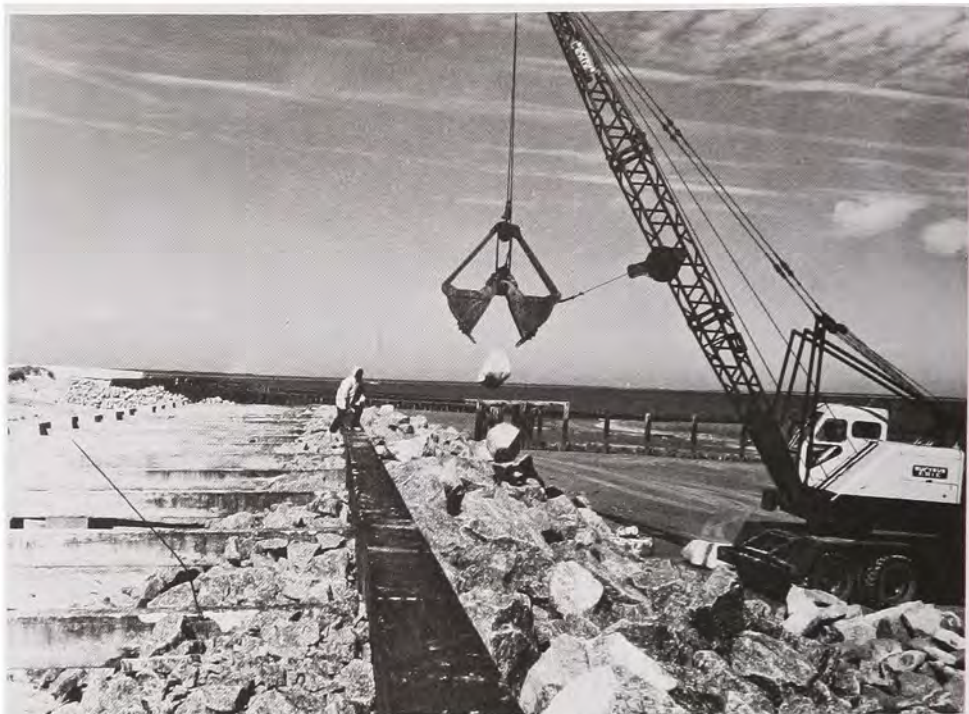
Hurricane damage repair being conducted on Tybee Island, Georgia following Hurricane Dora in 1964. February 1965. (Savannah District, Corps of Engineers)
