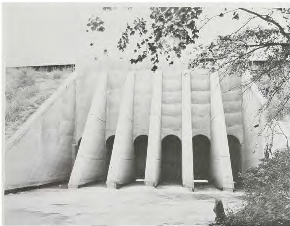
Sibley Mill Gates on the Augusta Levee as of 16 October 1940 following raising and strengthening of Wannamaker and Wells, Incorporated, under contract with the Corps of Engineers. (Savannah District, Corps of Engineers)
