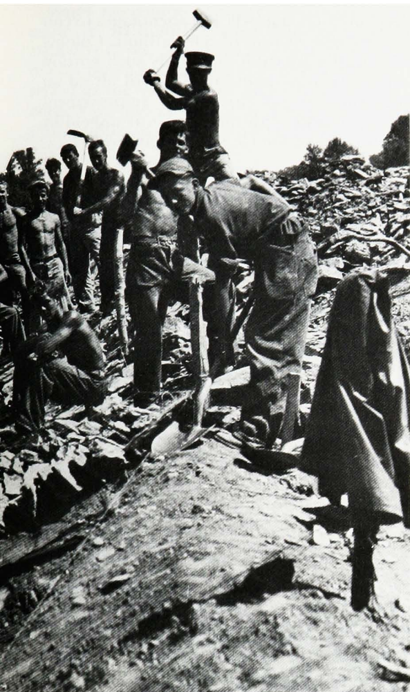
Wallkill River, New York, Flood Control Project Under Construction by Junior Civilian Conservation Corps Youths, 1936.
