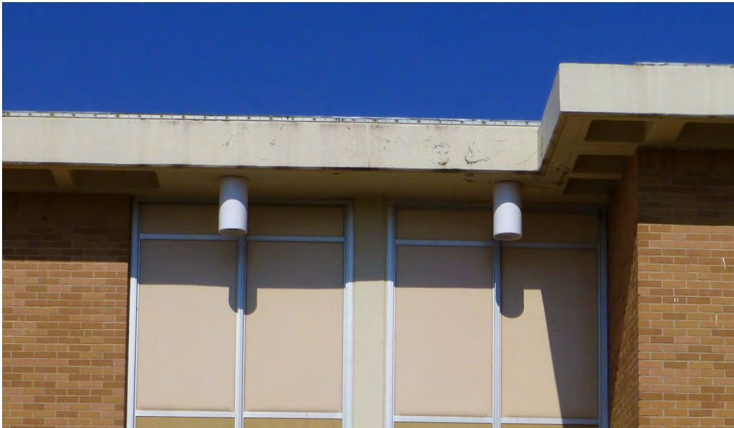
Figure 77. Ceiling-mounted light fixtures located under the concrete overhang at an entry bay on Building 29817, Allison Hall (ERDC-CERL, 2015).
