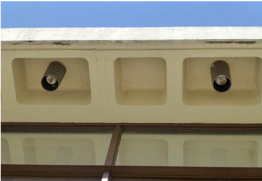
Figure 78. Ceiling-mounted light fixture placed within the concrete waffle overhang above an entry bay on Building 29818, Johnston Hall (ERDC-CERL, 2015).
