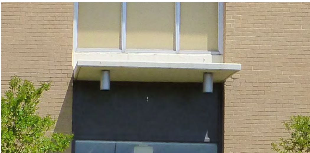
Figure 72. Ceiling-mounted light fixture placed on the underside of the flat concrete canopy, Building 29801, Nelson Hall (ERDC-CERL, 2015).
