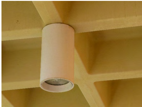
Ceiling-mounted light fixtures.
