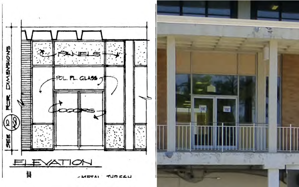
Figure 269. Entry bay for Building 29808, comparison of the original drawing detail from 1966 [left] to the current condition of the bright-aluminum and plate-glass doors and windows with insulated panels [right] (ERDC-CERL, 2015).
