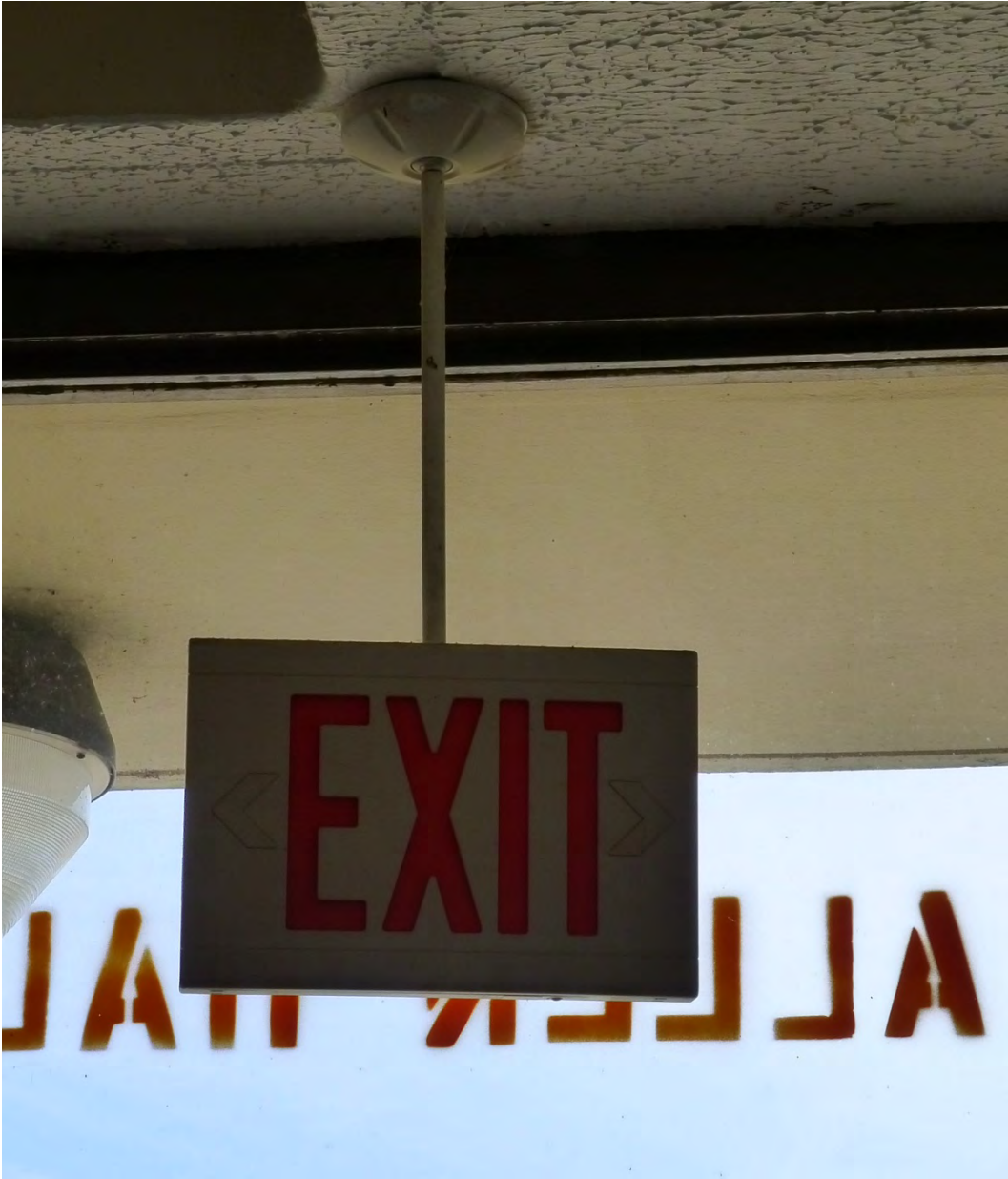
Figure 172. Typical suspended exit sign (ERDC-CERL 2015).
