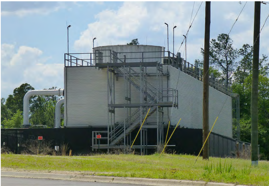
Figure 461. Building 25910 AC Cooling Towers, north of the Heating/AC Plant (ERDC-CERL, 2015).
