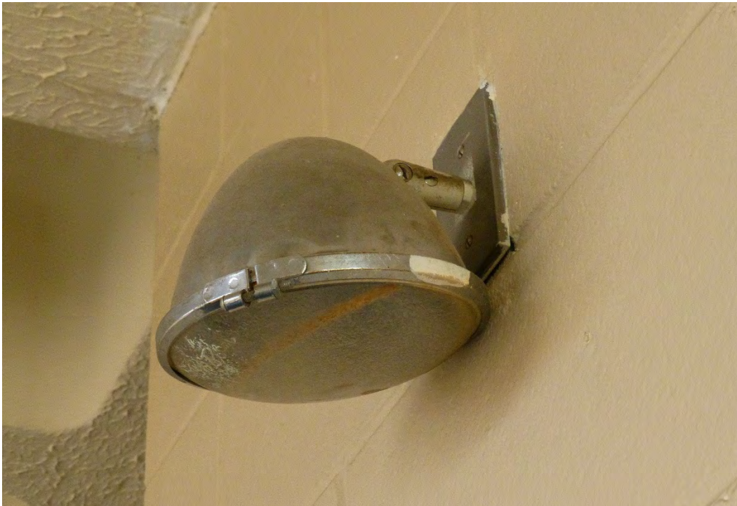
Figure 141. Original interior wall-mounted light fixture located in a stairwell (ERDC-CERL, 2015).
