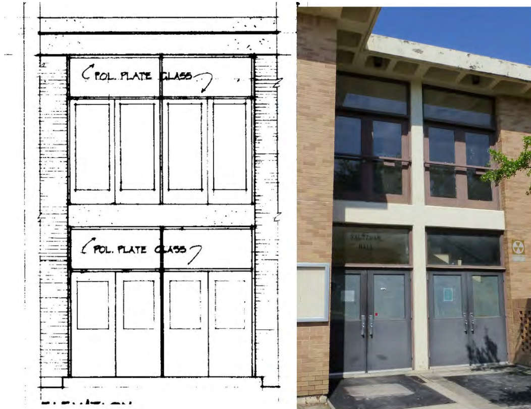
Figure 294. Doors on the east and west elevations – comparison of the original design and materials from 1964 [left] to the current condition of the metal doors with pane and transoms on the first floor and the metal and plate-glass doors with security bars on the second floor [right] (ERDC-CERL, 2015).
