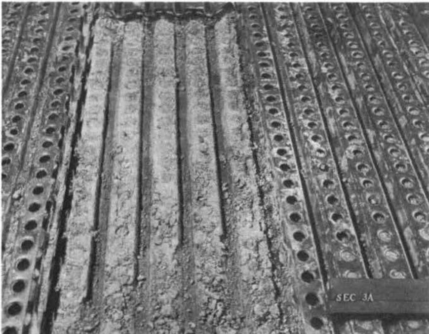
Fig. 2. Appearance of subgrade after removal of plank at 528 coverages
