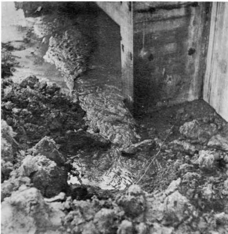
Large boil along east side of conduits at monolith 7 (12 Dec 1951)
