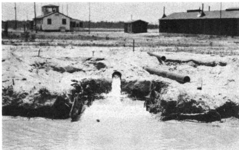
6-in. pipe discharging into sump for ponded area
