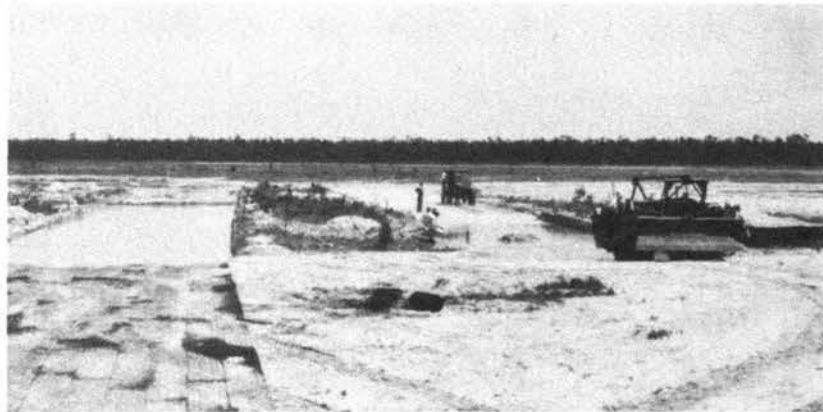
Beginning tracking with 80,000-lb tractor, Section 4 Ditch between Sect.3 & 4 left, both ponded areas flooded
