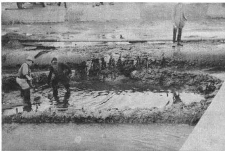
Fig. 2. Typical damage to stilling basin steps
