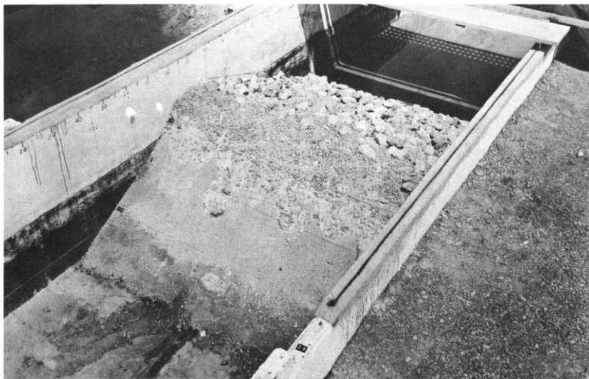
Fig. 10. Crest of rock fill after stability tests of the seal cover. Note loss of seal cover near the crest
