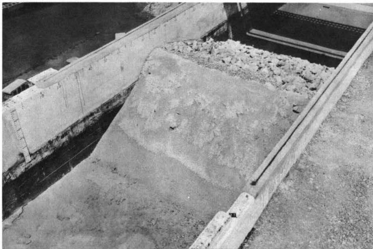
Fig. 8. Completed seal cover placed on top of the riprap blanket on upstream slope of fill
