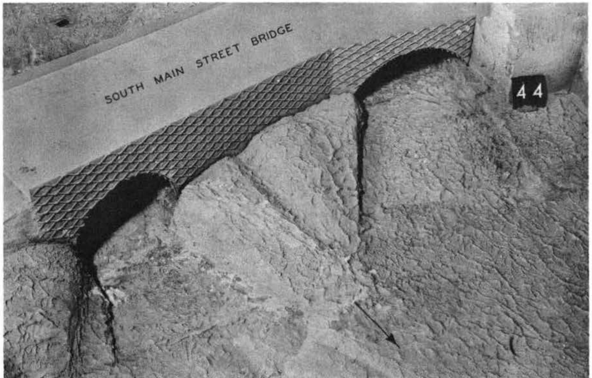
Photograph 18. Plan B: Rock excavation on left side of channel below the west arch of the South Main Street bridge with flare reduced to 10 degrees
