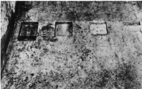
Fig. 11. Test recesses in floor of conduit, looking upstream, after one month's intermittent operation
