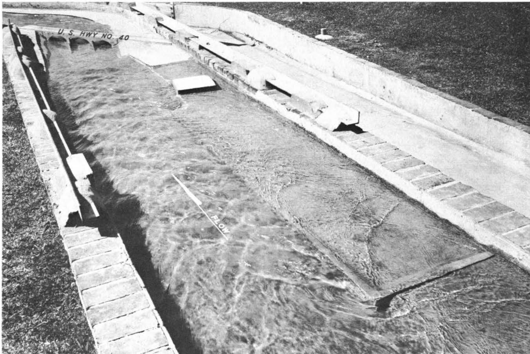
Photograph 13. Flow conditions above U. S. Highway 40 bridge (note flooding of right overbank). Discharge: Wills Creek, 50,000 cfs; North Branch, 63,000 cfs
