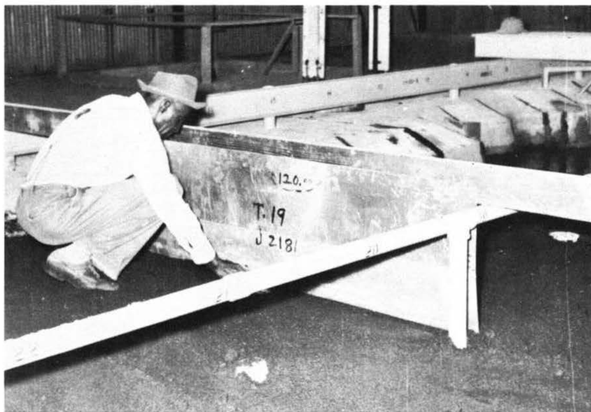
Fig. 7. View of bed molding operation using sheet-metal templates suspended from graded rails
