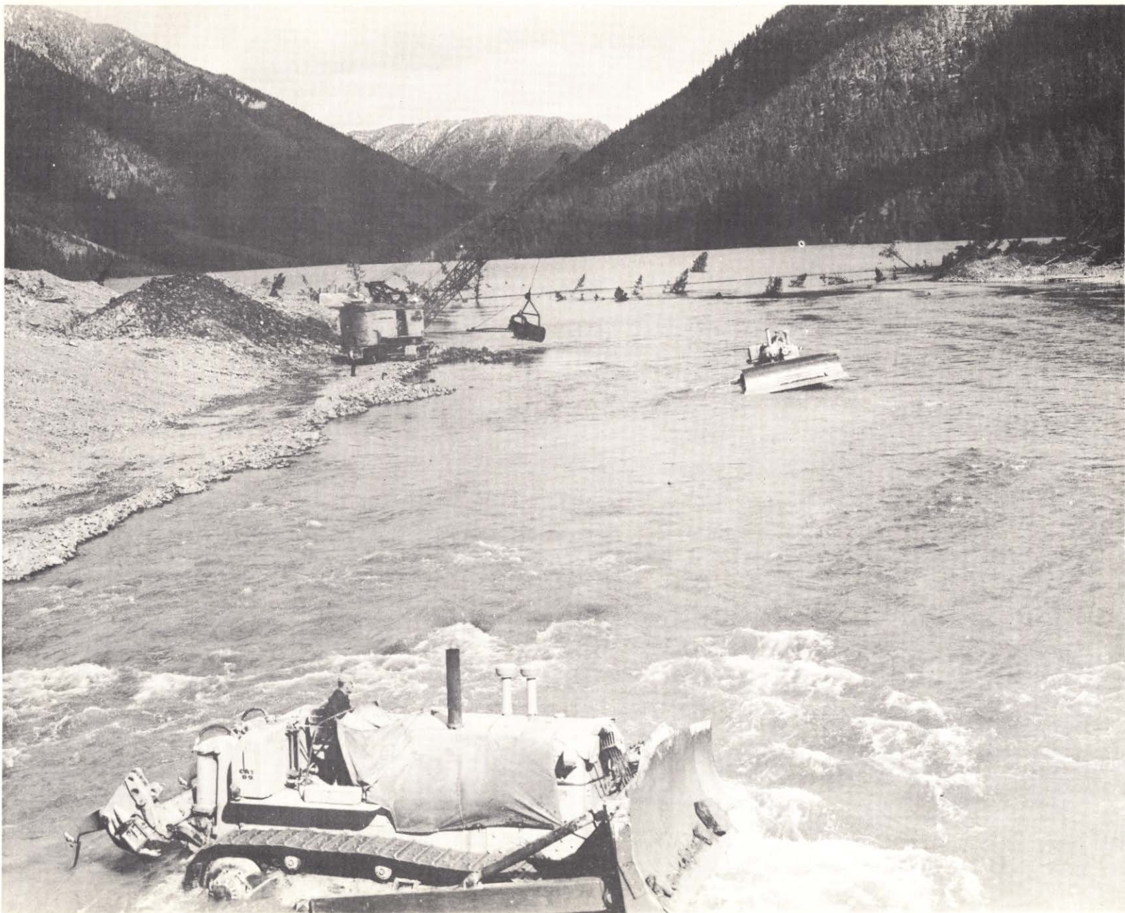
Photo 15. 29 September 1959. Starting to lower the spillway channel near the outlet of Earthquake Lake.
