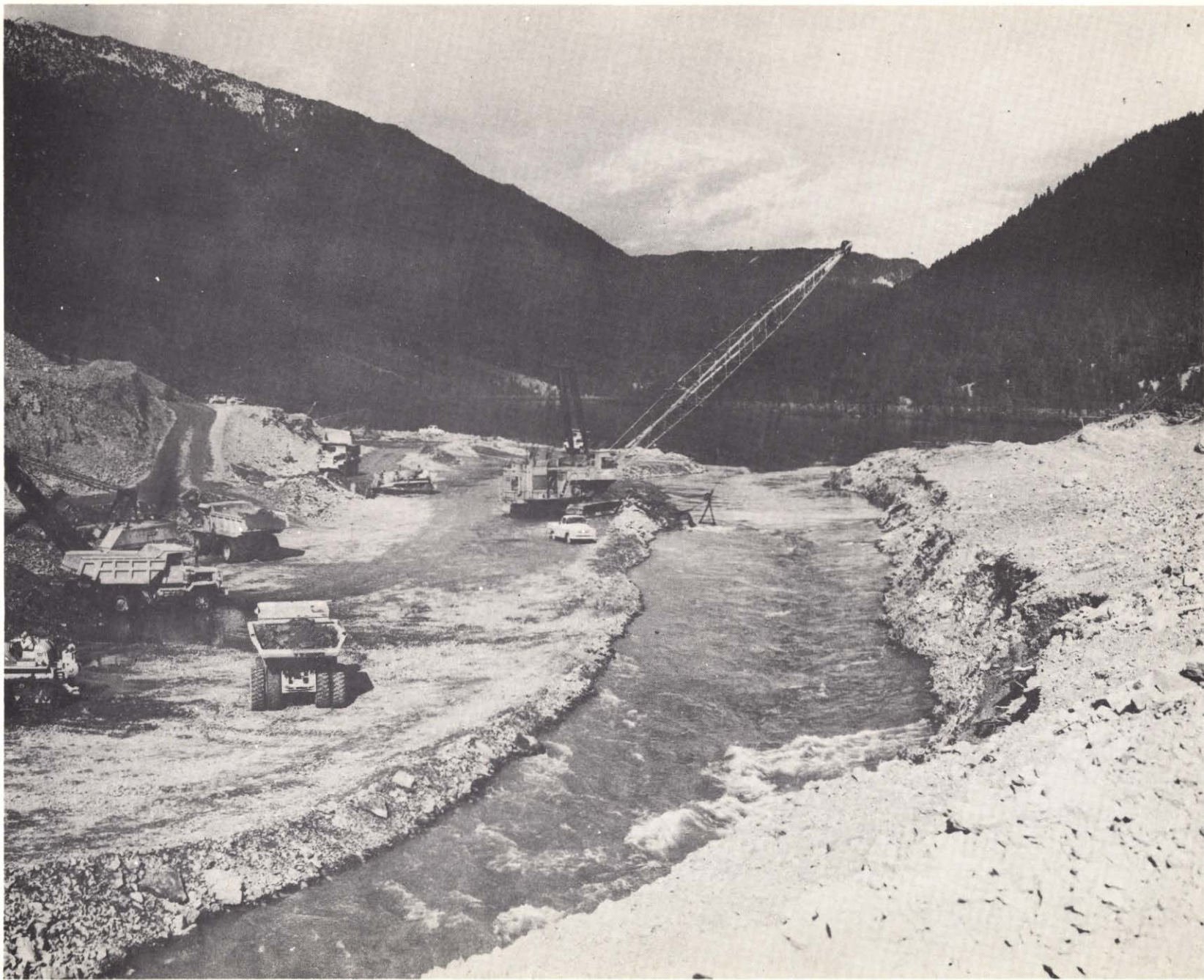
Photo 21. 11 October 1959. Large dragline lowering spillway channel near the outlet of Earthquake Lake.
