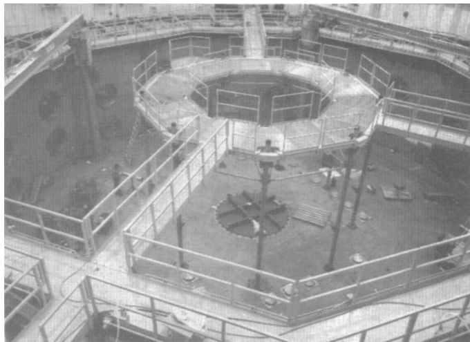
Figure 3. Accelerator tank with center-section work platform.
