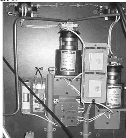
Figure 6. D Size Ignitron / Trigger System
