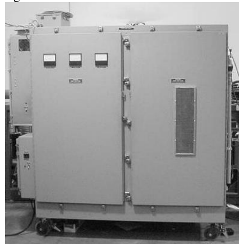
Figure2. Pulsed Power Enclosure Photo © Maxwell
