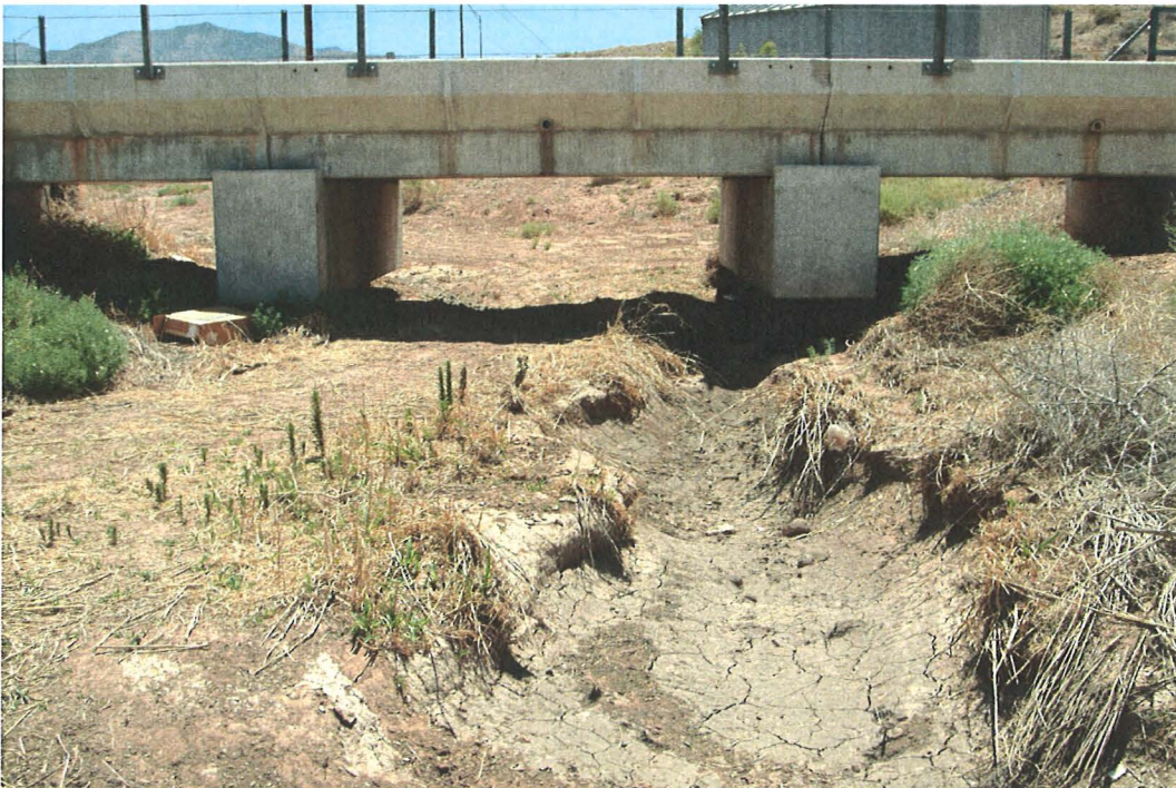
Photo 10. A downstream view of the same drainage feature in the previous photo (70°).
