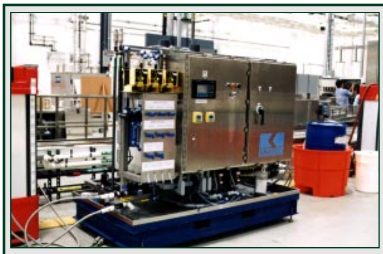
Reverse Osmosis Purification System
