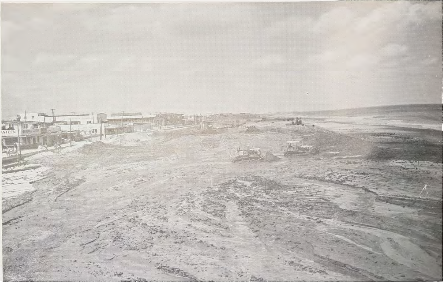
Carolina Beach berm and dune was constructed in 1965. View shows work in the boardwalk area.
