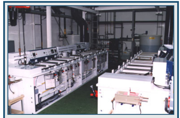
Closed-Loop Manual Plating Line
