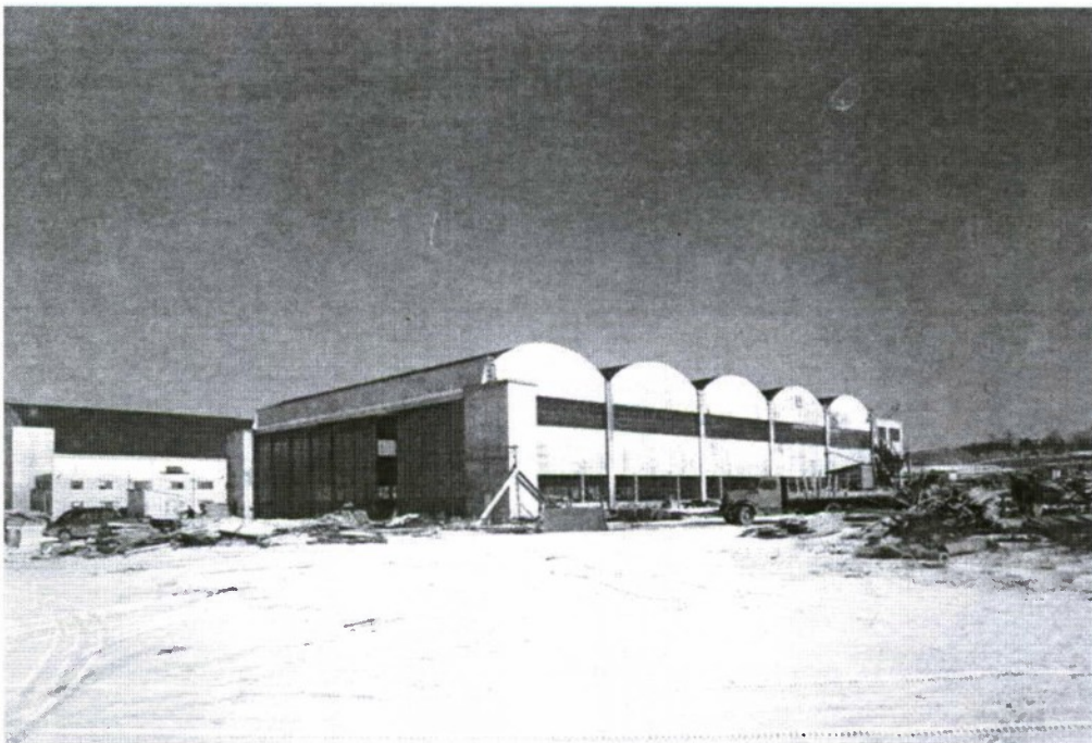
Plate 4: Anton Tedesko (Roberts & Schaefer). Signal Corps Hangar (Building 20006), Wright Field. Under construction, 11 January 1943. Courtesy of the History Office, 88 th Air Base Wing, Wright-Patterson Air Force Base.
