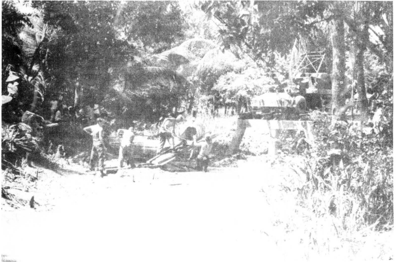
Members of Seabee Team 1009 prepare a concrete foundation for a foot bridge in a hamlet west of Vinh Long.
