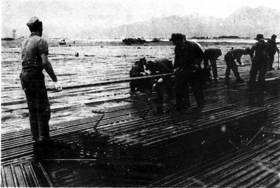
Seabees prepare to place a section of matting at the Helicopter Maintenance Facility for the 1st Air Cavalry at Red Beach.
