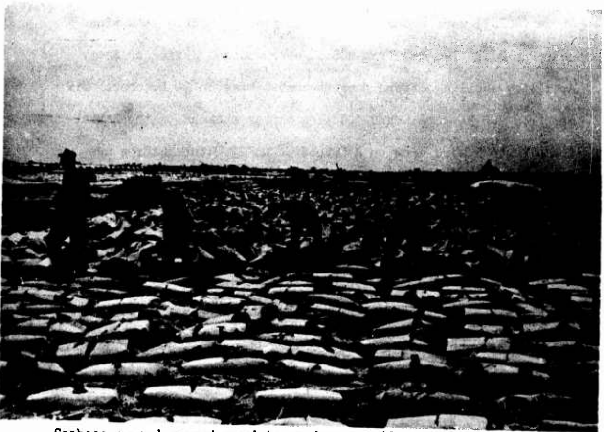
Seabees spread cement used to produce a soil base for the new airstrip at Dong Ha.
