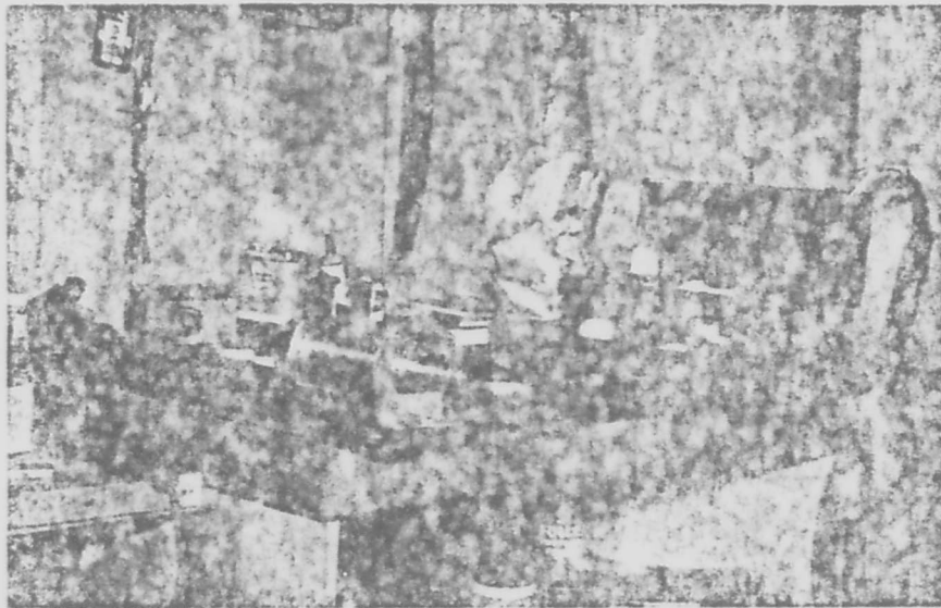
Figure 2.4 Modified Mark VIII transducer attached to armored submarine cable. Note: Splice has not been waterproofed.
