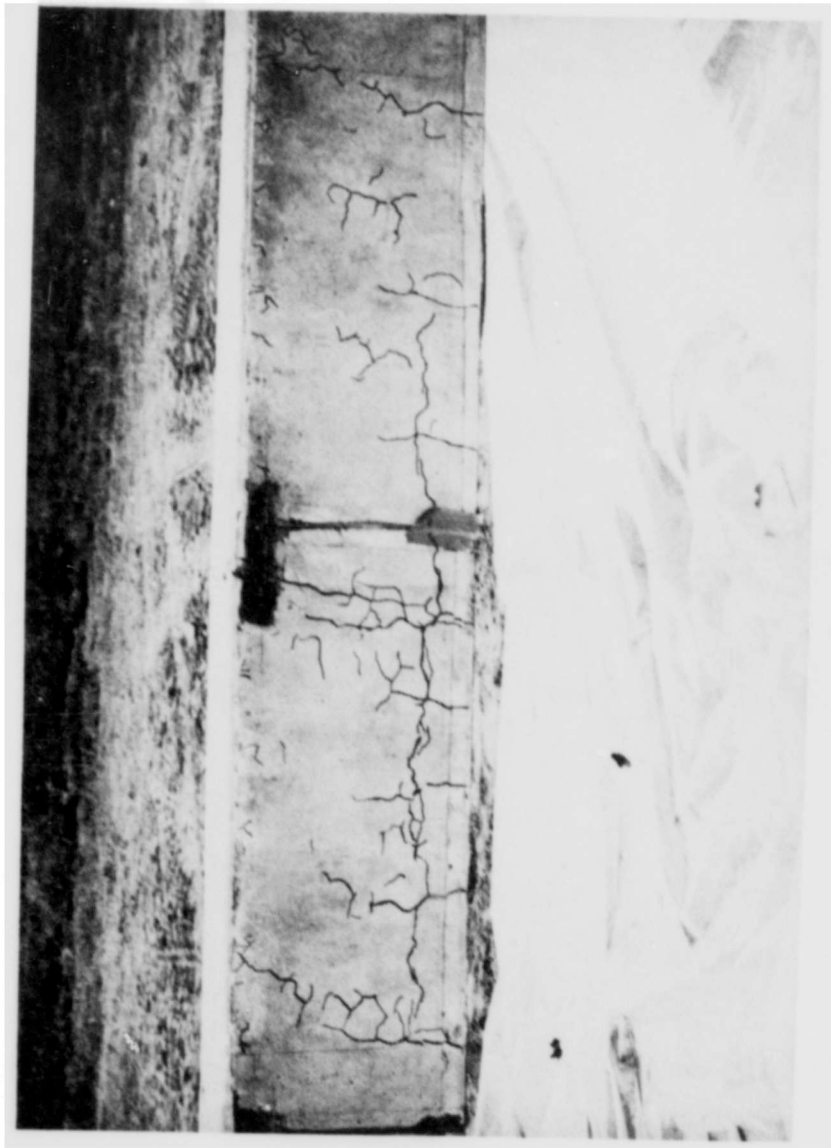
Figure 28. Side View of Beam 3 After Test No. 4
