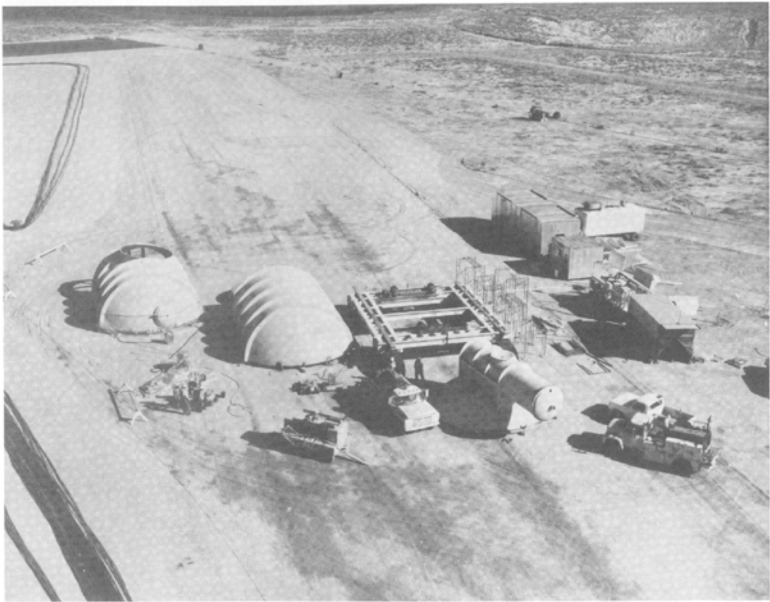
Figure 7.2 HURON KING event - major components of the experiment tank prior to assembly.
