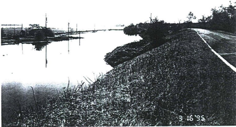
IN 1995, POND CREATED FROM EXTENSIVE SEEPAGE ALONG LEVEE TOE AT SITE 18, FEATHER RIVER/YOLO BYPASS. LAST TIME WATER PONDED HERE WAS IN 1985.
